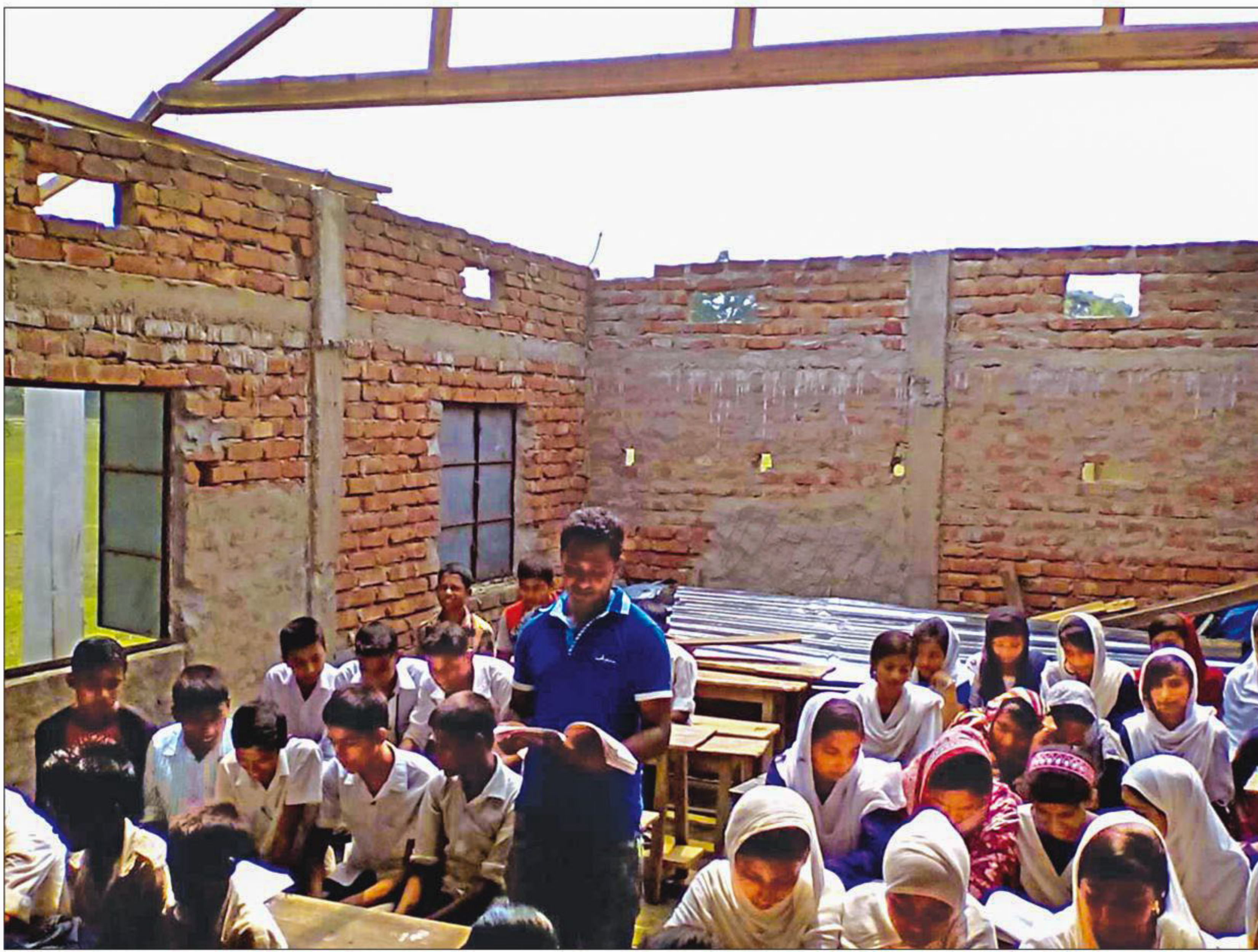
Class-VI students sit in their room that has no roof. A nor'wester blew away the roof of Monohorpur High School in Kulaura of Moulvibazar on April 22. The school has been running only on sunny days since then.
