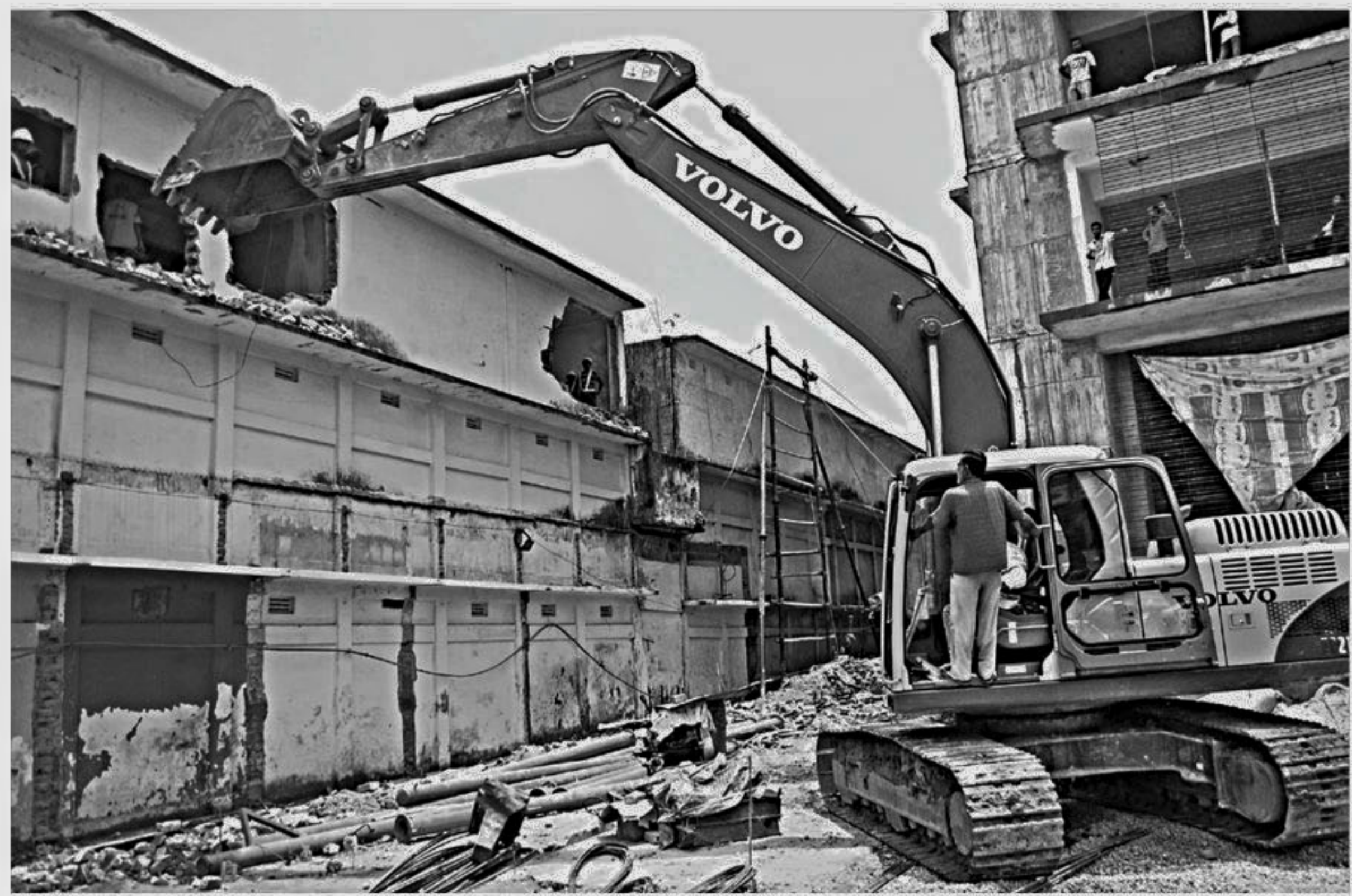
Sylhet City Corporation bulldozing a portion of the risky City Super Market building yesterday. This three-storey structure is one of 32 residential and commercial buildings vulnerable to earthquakes. Earlier on April 21 and May 8, two buildings were demolished. PHOTO: SHEIKH NASIR
