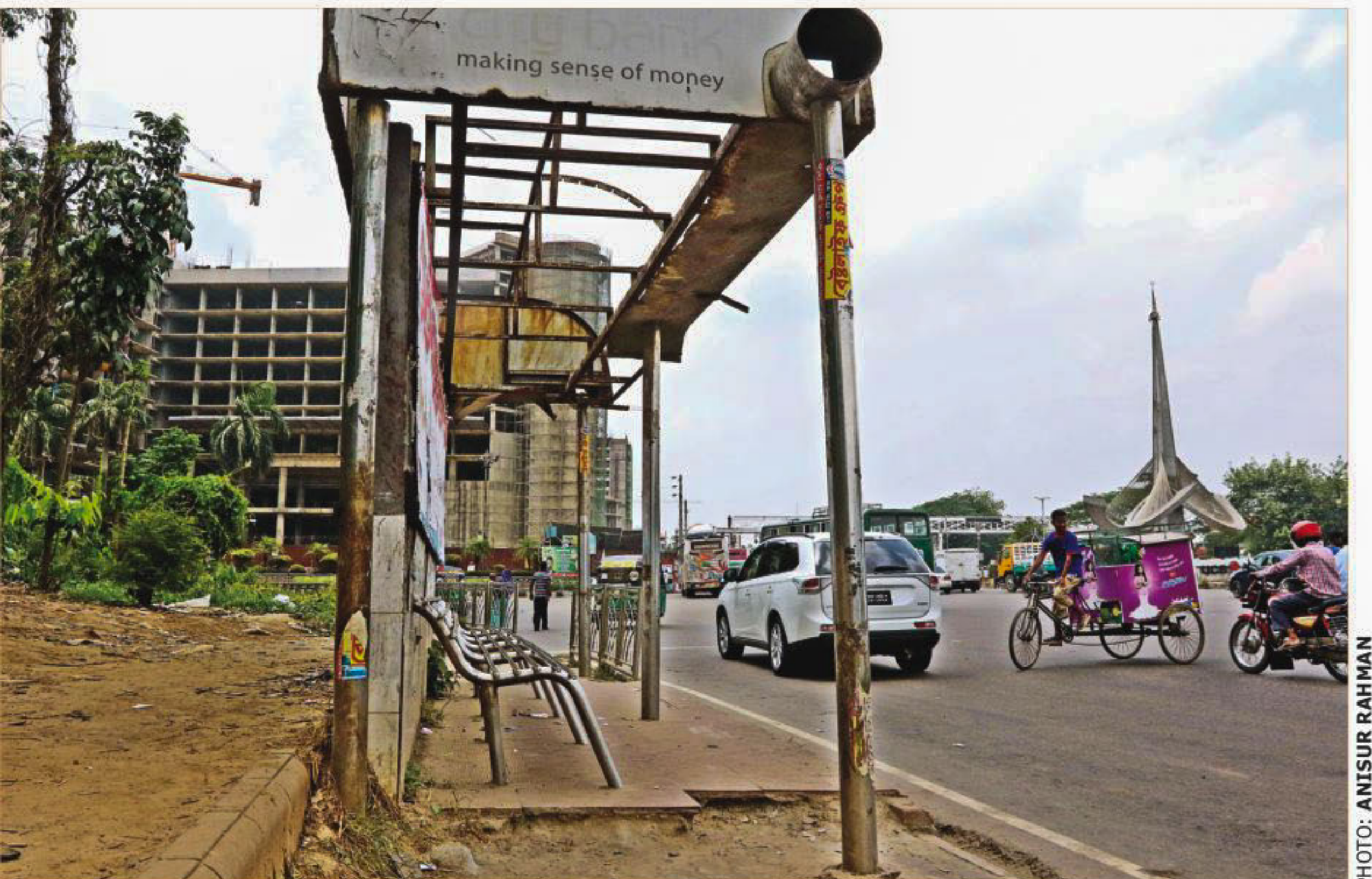
A passenger shade on the entrance road to Hazrat Shahjalal International Airport is in extremely bad shape. Even the shade overhead to protect passengers from the sun or rain is gone. The photo was taken a few days ago.
