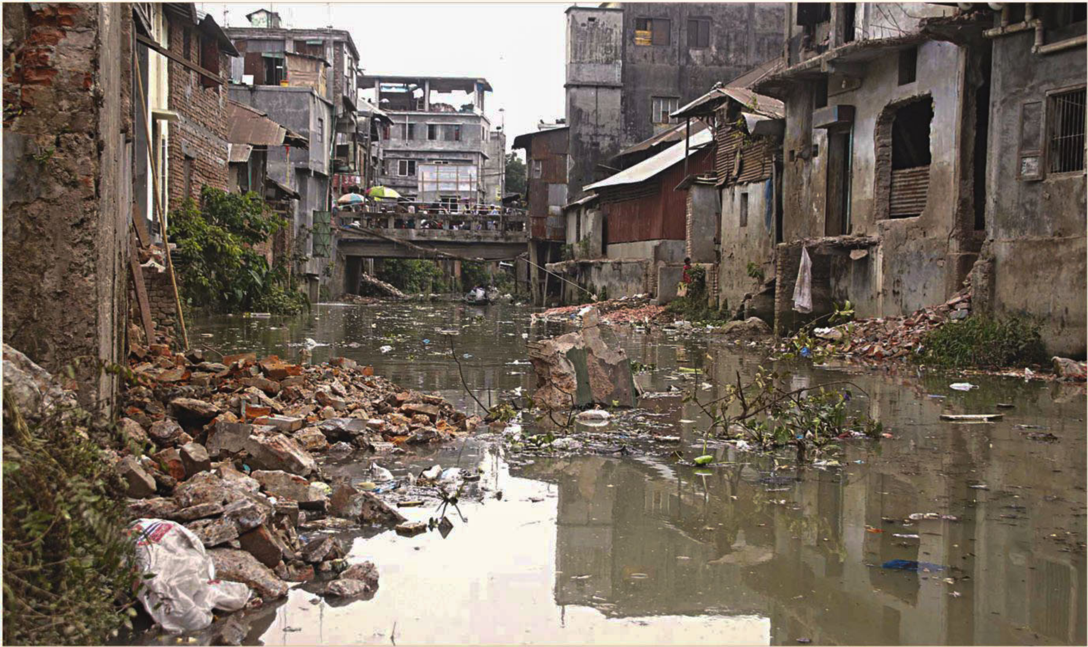
Rubbles block Jail Khal in Barisal city since the district administration's demolition drive on its banks 10 days ago, hampering transport of commodities by trawlers through the canal connected to the Kirton Khola river. This 2km canal is the only route for carrying goods to and from Chawkbazar wholesale market, says our Jhalakathi correspondent. The authorities said they would remove the concrete and dredge the canal after finishing the drive but did not say when. The photo was taken yesterday.
