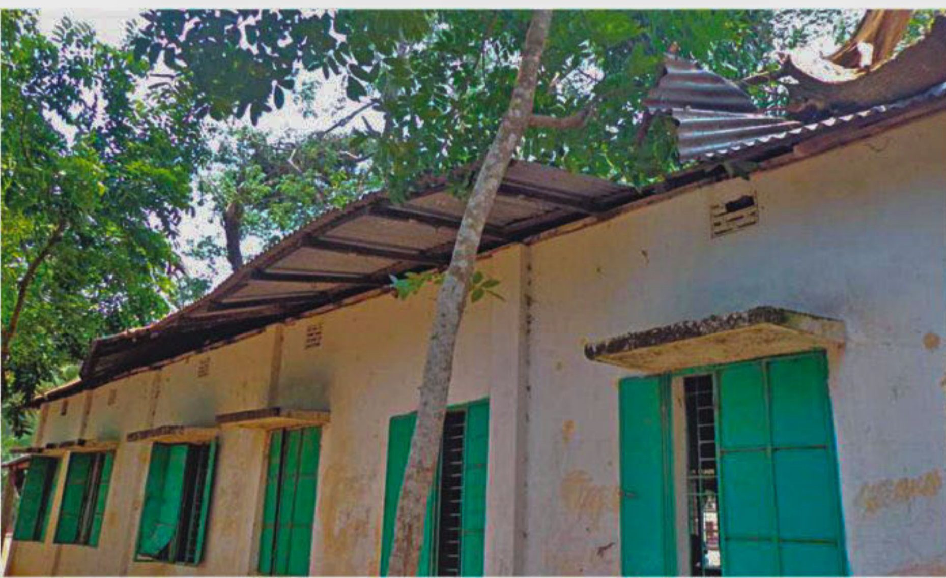
PHOTO: STAR Storm-damaged Medila Adarsha High School in Bhaluka upazila under Mymensingh district.
