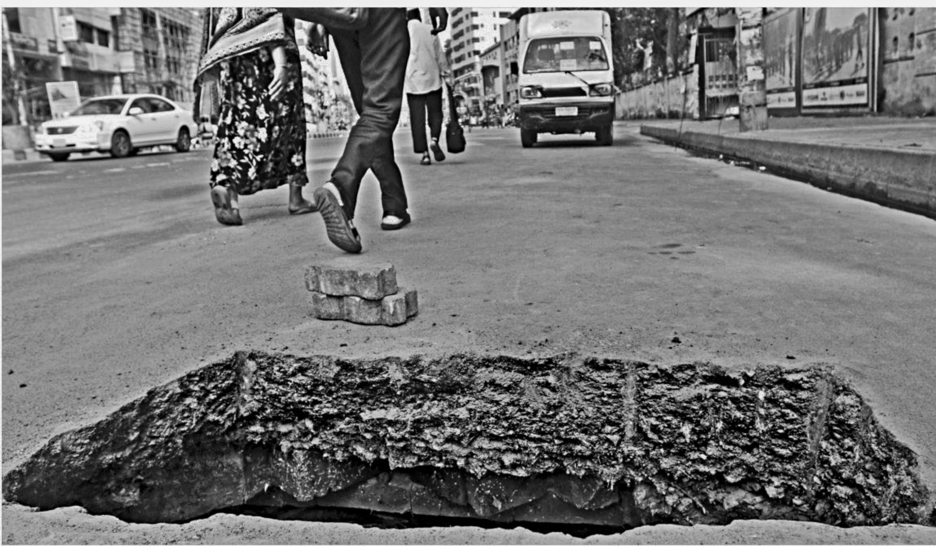
Just another day in the capital! A sizable hole dug up around 25 days ago in order to repair a gas line might be seen during the daylight, but dangers mount as night falls in front of the capital's Paltan Model Police Station, is another reminder of where are the authorities concerned when you need them. The photo was taken yesterday.
