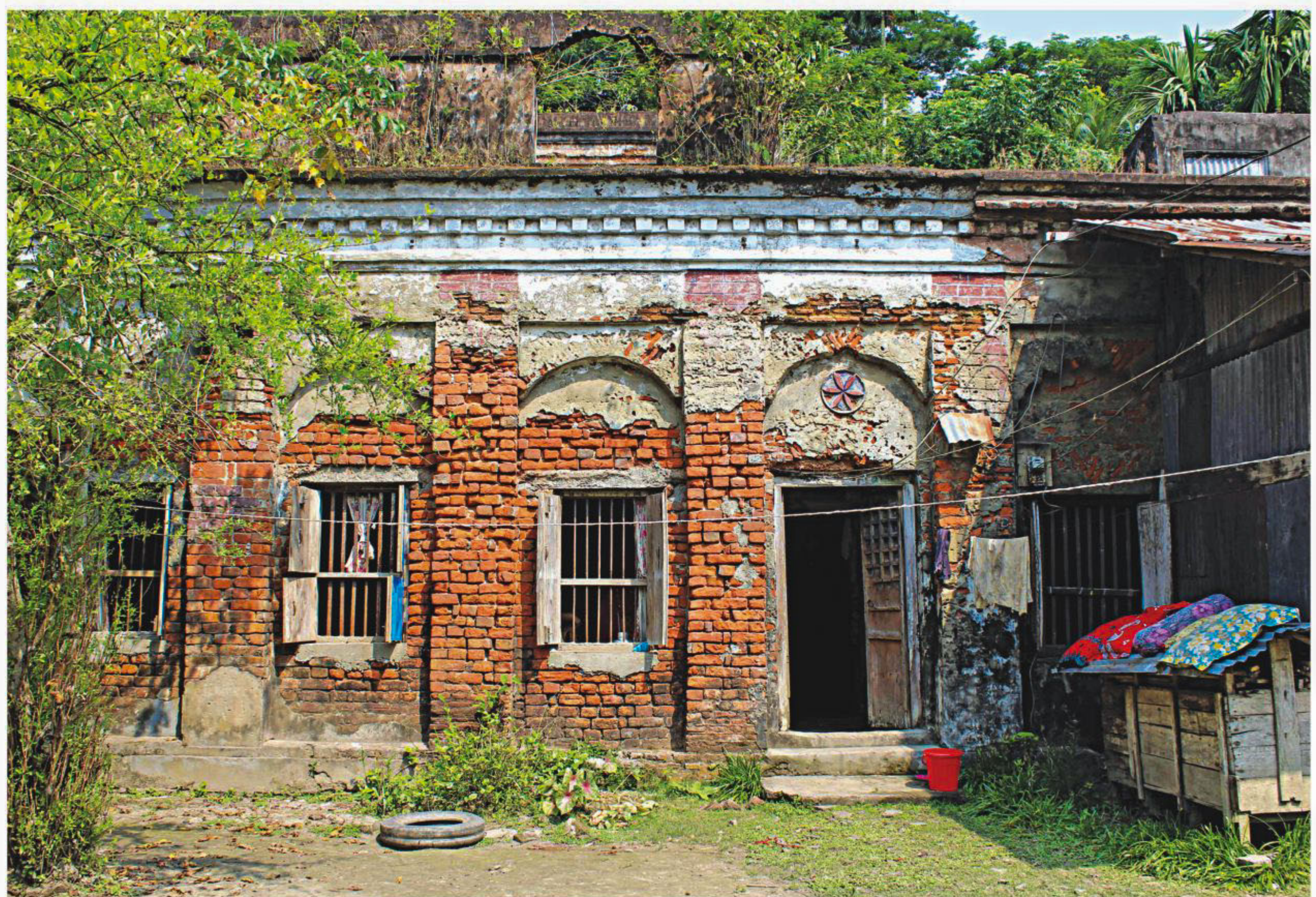
Tourists still come to see the home at Satura village of Rajapur upazila in Jhalokathi where Sher-e-Bangla A K Fazlul Haque was born 142 years ago. The single storey British Raj era building is in a decrepit state as no authority cares enough to look after it. The photo was taken recently.
