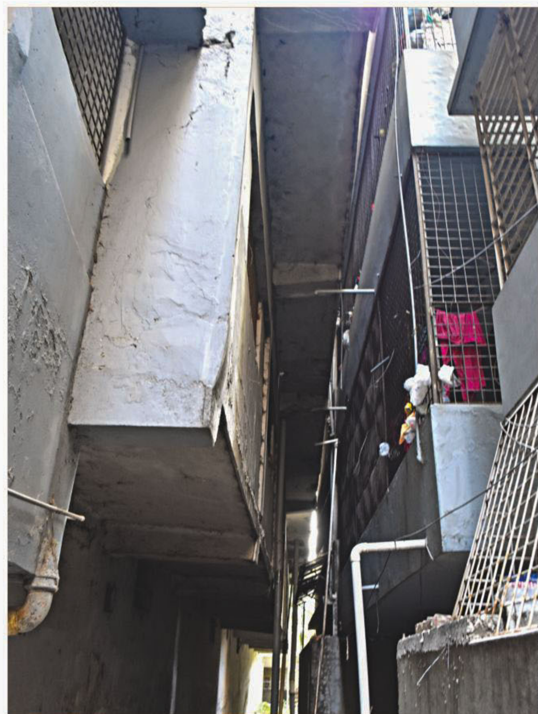
The RMG factory building, left, that tilted on an adjoining residential one in the capital's Tejgaon area on Monday; forces us to ask why a factory building be allowed to function next to a residential one or set up in the inhabited areas of municipalities?
