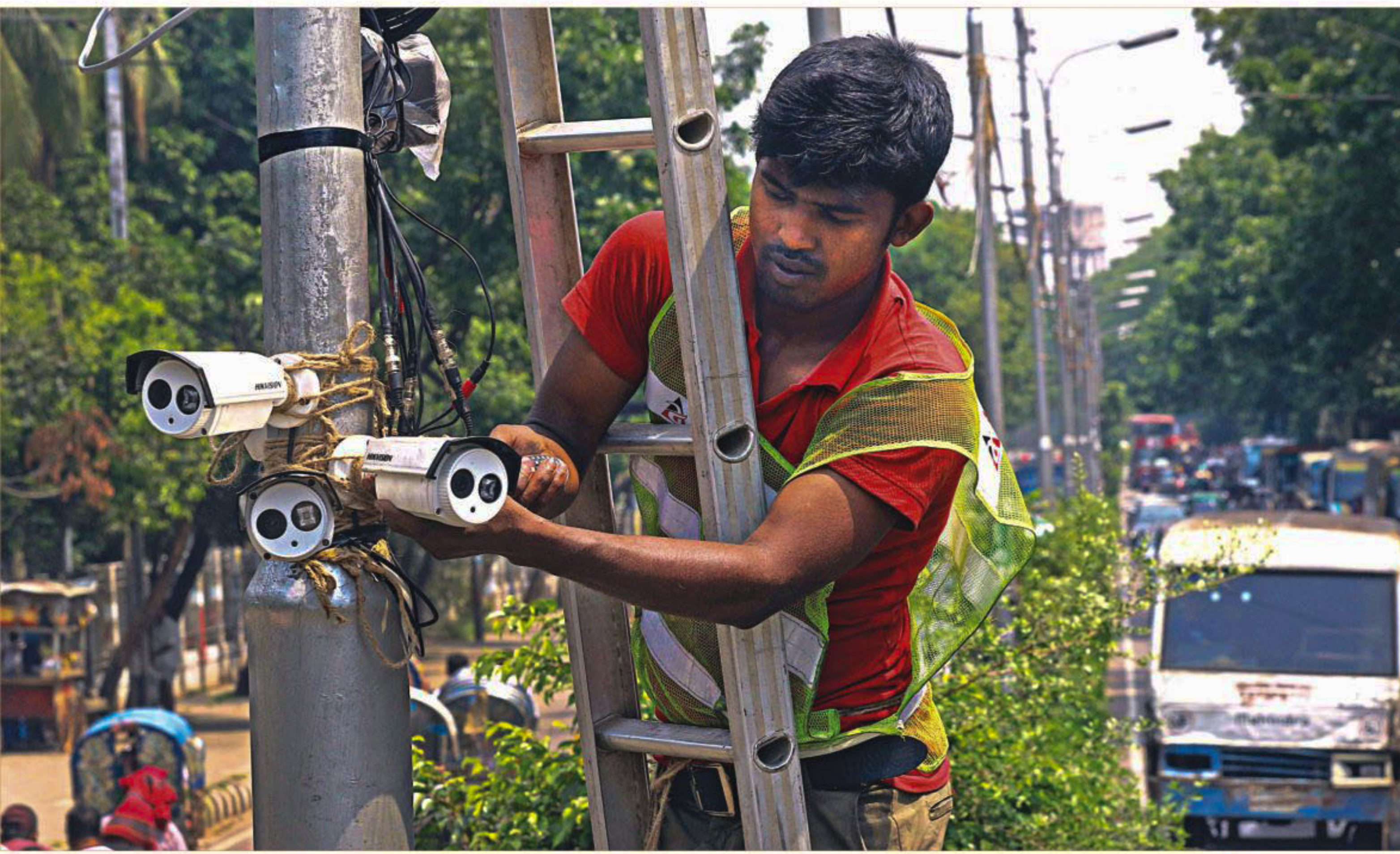
CCTV cameras being set up in front of TSC of Dhaka University yesterday as part of the authorities' move to bring the entire area under scanner ahead of Pahela Baishakh, the first day of Bangla calendar.
