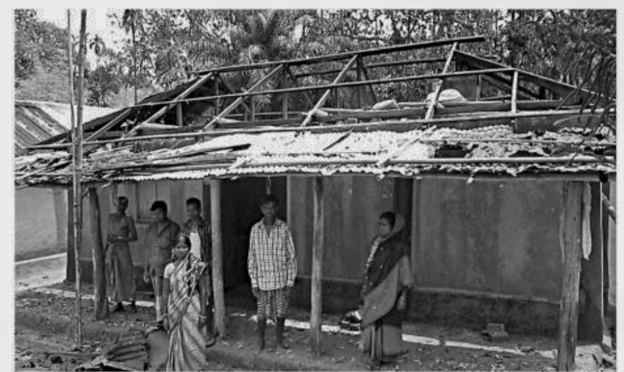
Like many others, a house at Lakkhichhara Tea Garden in Barlekha upazila under Moulvibazar district lies ravaged as a hailstorm lashed the area Friday night.
