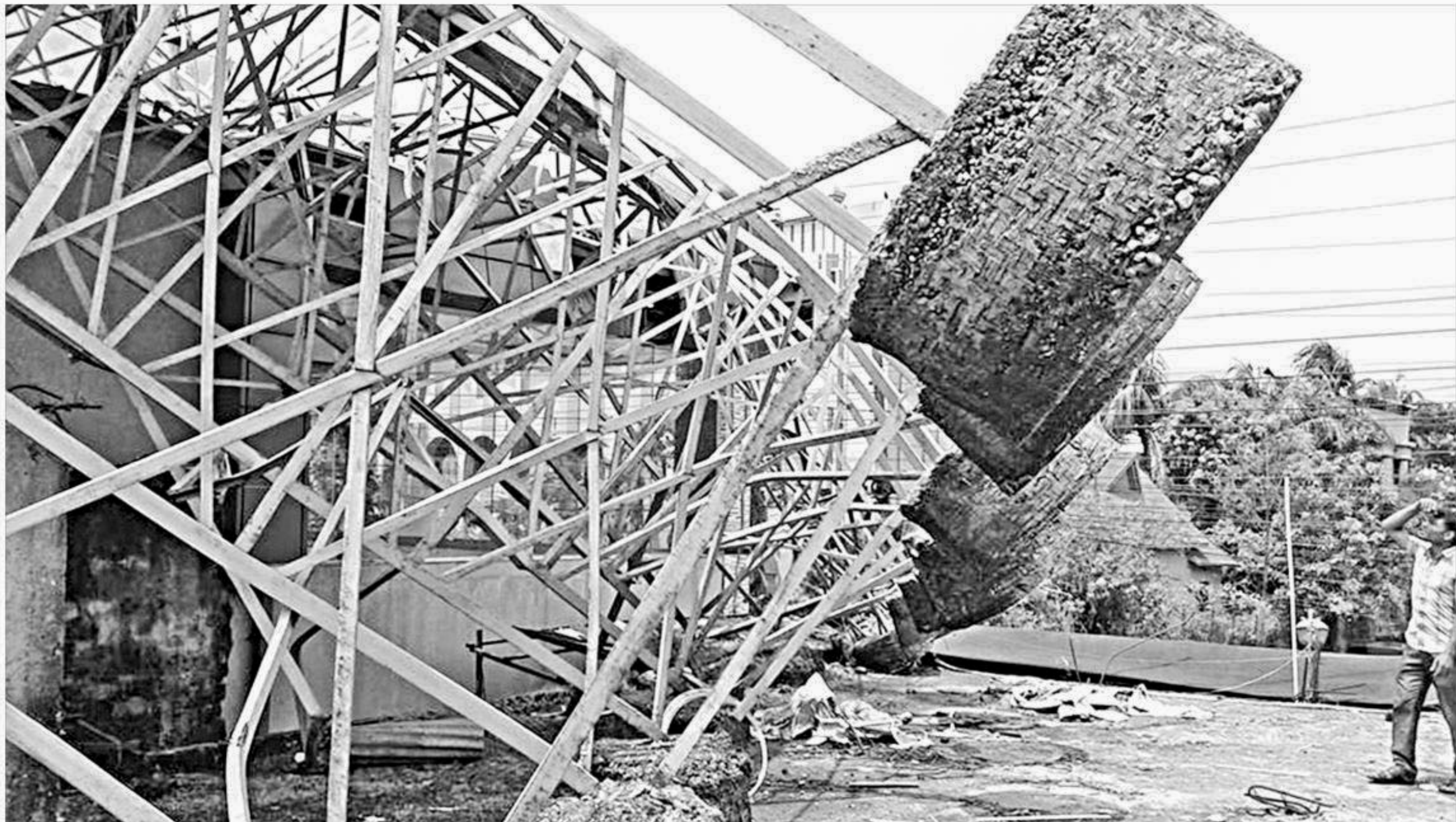
A rooftop billboard collapsed in Sylhet city's Nairpur area during Wednesday night's storm. Many of the city's billboards are erected illegally on flimsy structures and without proper safety measures, which can cause serious accidents any time. Locals continue to urge the authorities concerned to dismantle these hazardous billboards, which keep mushrooming due to their indifference. PHOTO: STAR
