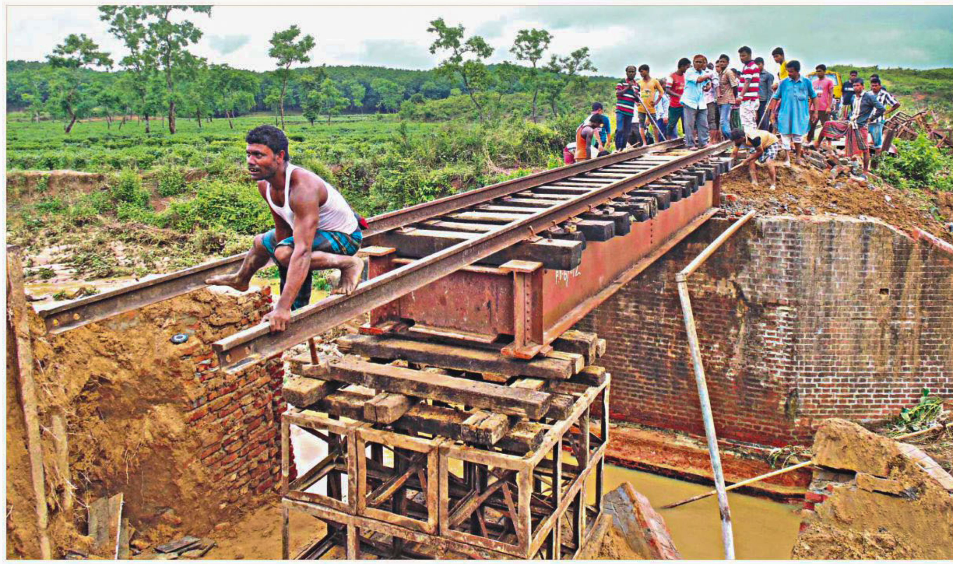
Workers repairing Jankichhora Railway Bridge on Akhaura-Sylhet route in Srimongol. The bridge subsided following heavy rains and flash floods, snapping rail communications between Sylhet and other parts of the country for hours yesterday.
