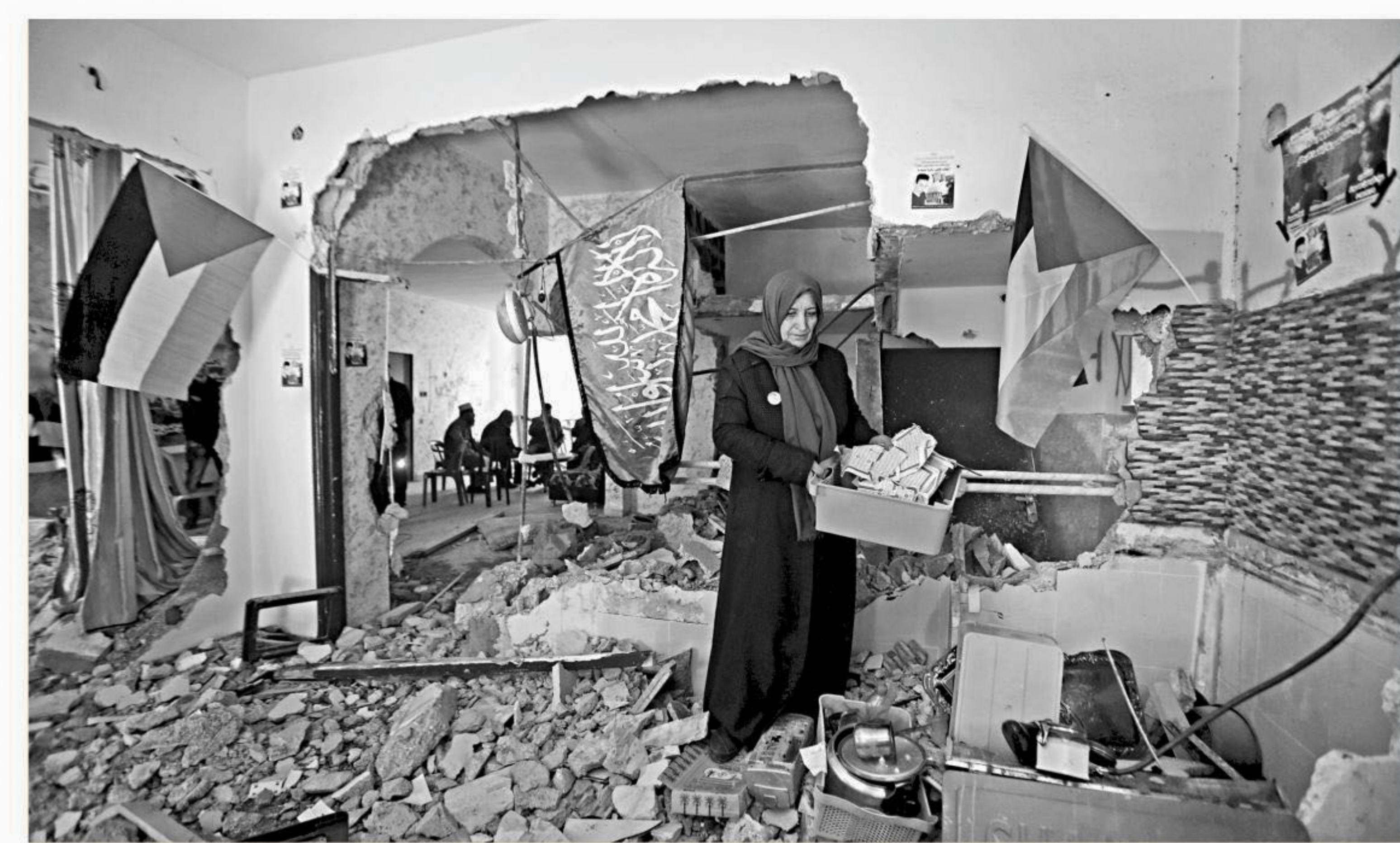
The mother of Palestinian Ihab Maswadeh inspects belongings after their family house was partially demolished by the Israeli forces in the West Bank city of Hebron, yesterday. According to the Israeli military, Ihab Maswadeh was shot dead by Israeli troops after he attempted to stab an Israeli soldier last December.
