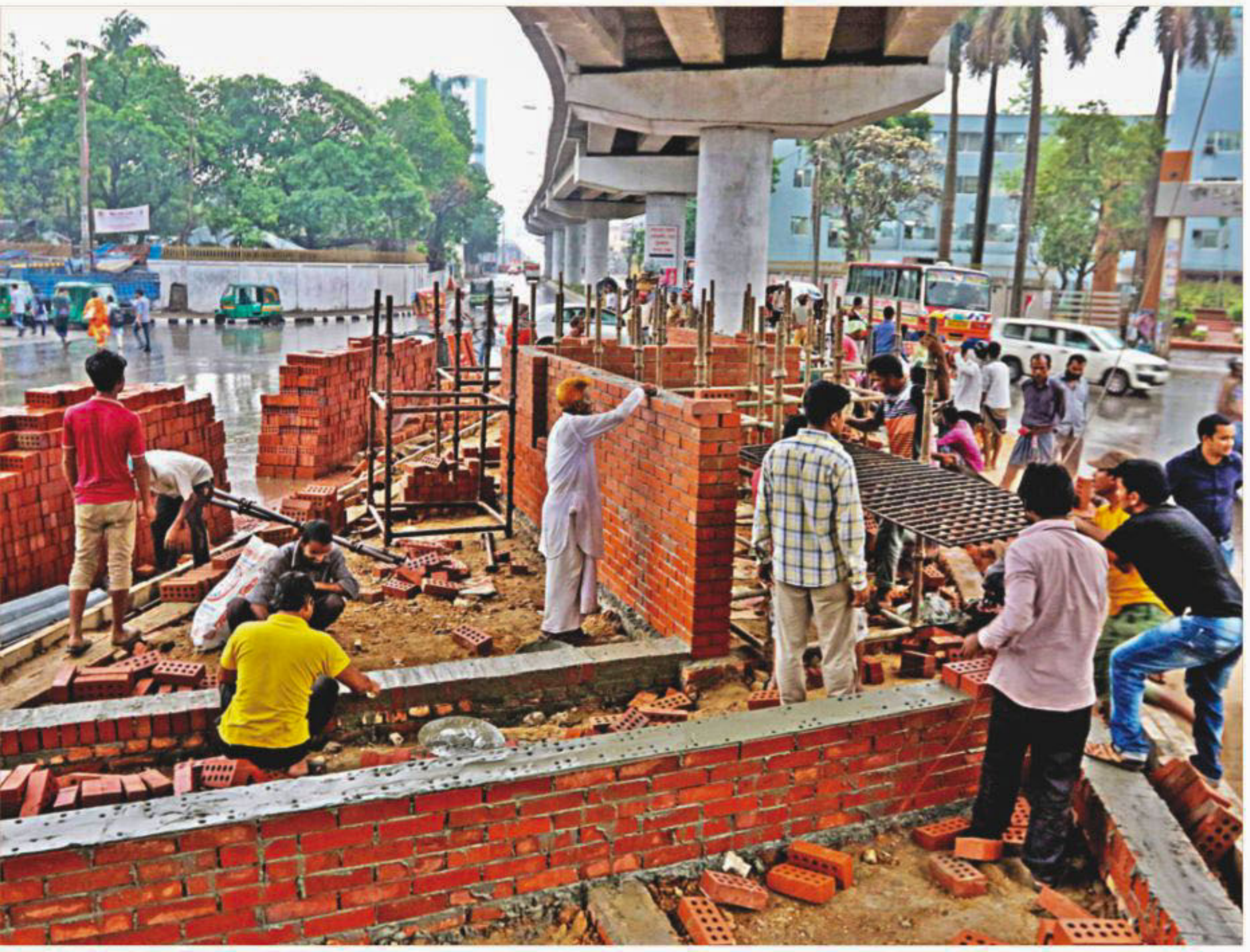
Workers busy constructing a median strip where the inauguration plaque of the Mouchak-Moghbazar flyover will be placed at the capital's Saat Rasta intersection. PHOTO: ANISUR RAHMAN
