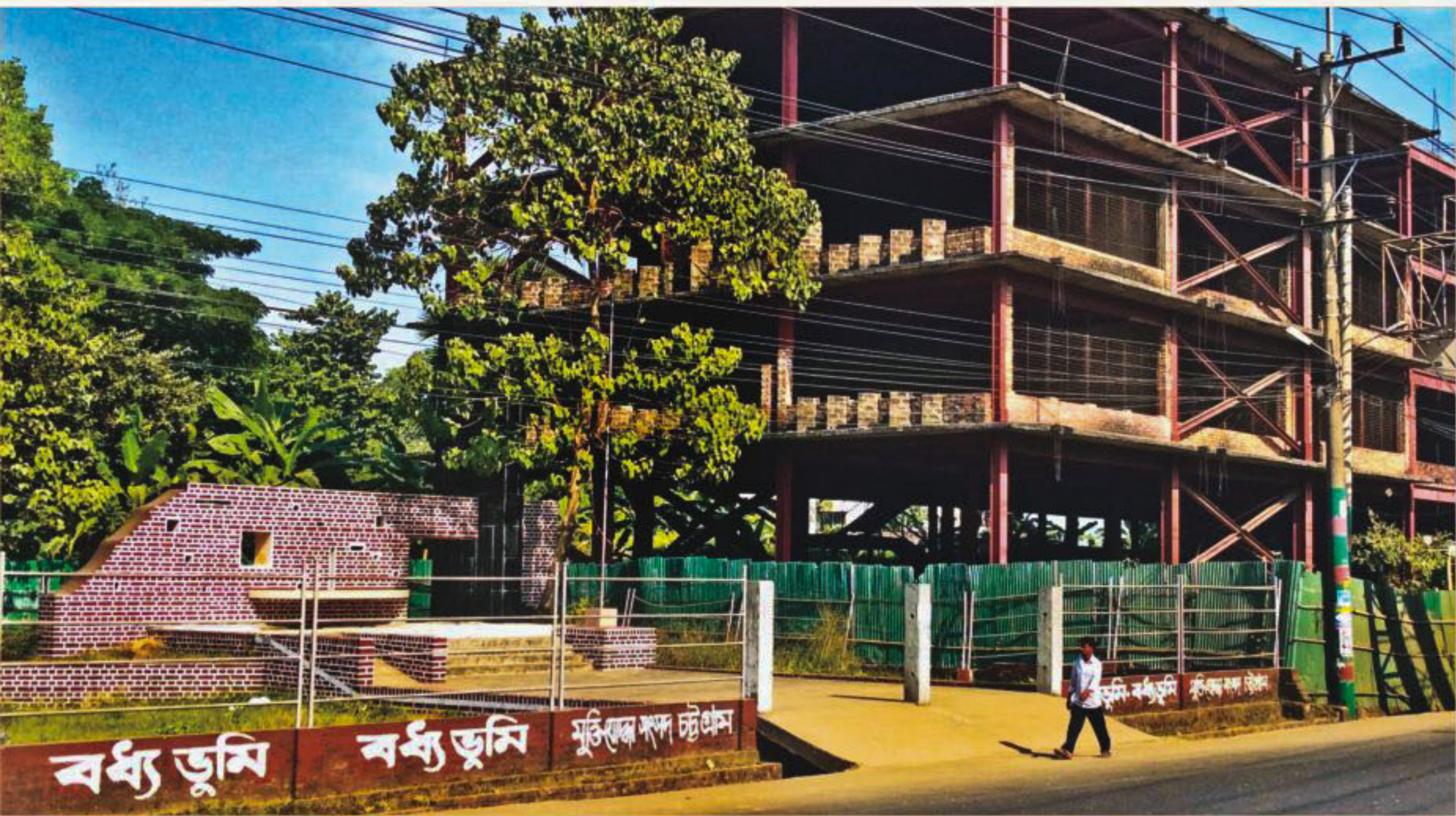
A four-storey building being constructed by the University of Science and Technology Chittagong (USTC) on a place in Pahartali of Chittagong, which is one of the largest killing fields in the country. Around 11,000 human skulls were found there, and the Supreme Court ordered the preservation of the entire 1.75 acre land as a killing field, but to no avail. USTC bought the private land, but amid public outcry donated 0.10 acres to build a small monument to mark the site as a killing field. The photo was taken on Thursday. PHOTO: ANURUP KANTI DAS
