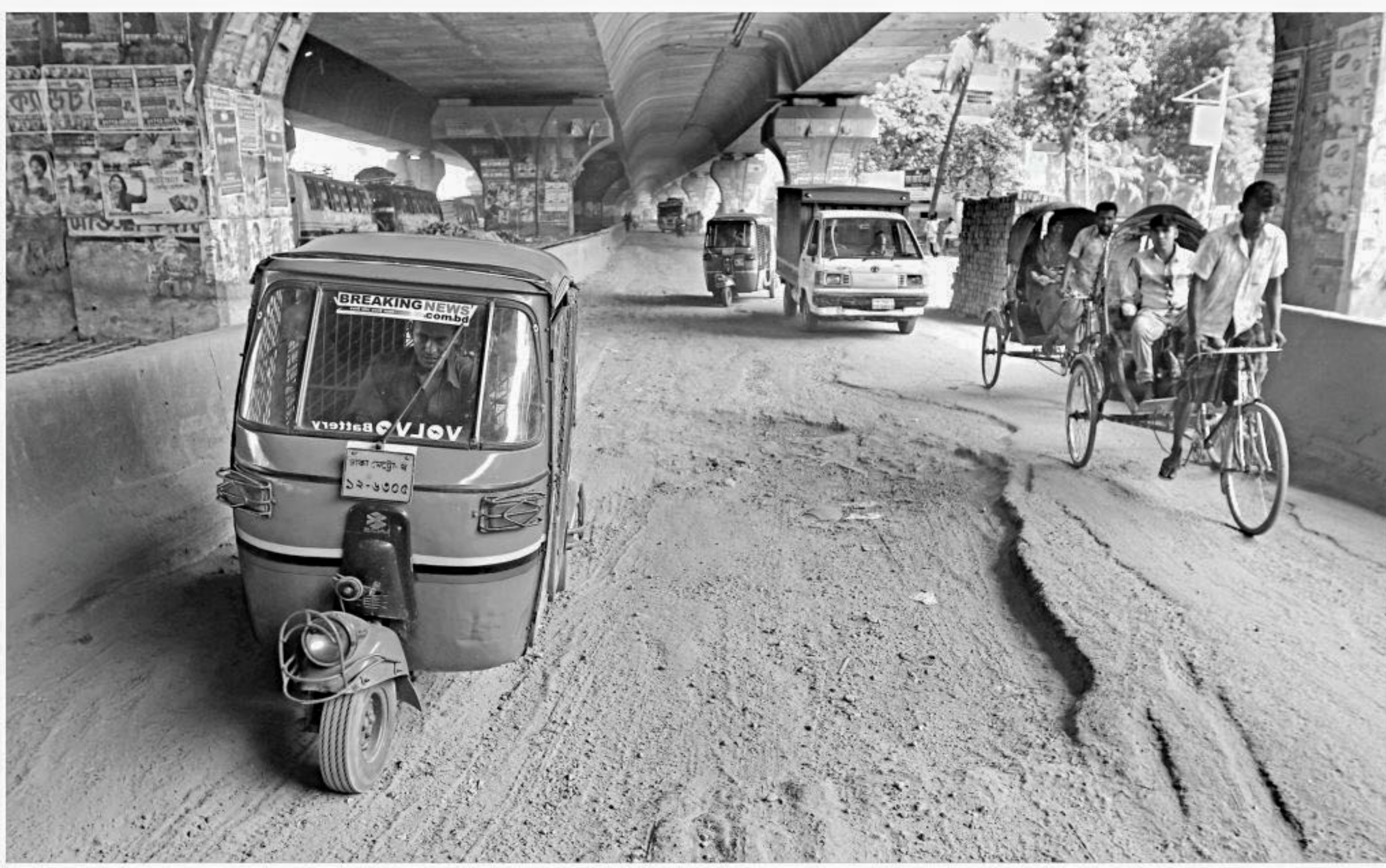
This road beneath Mayor Mohammad Hanif Flyover in the capital's North Jatrabari has been in a dilapidated condition for a long time, hampering vehicular movement. The photo was taken on Thursday. PHOTO: PALASH KHAN
