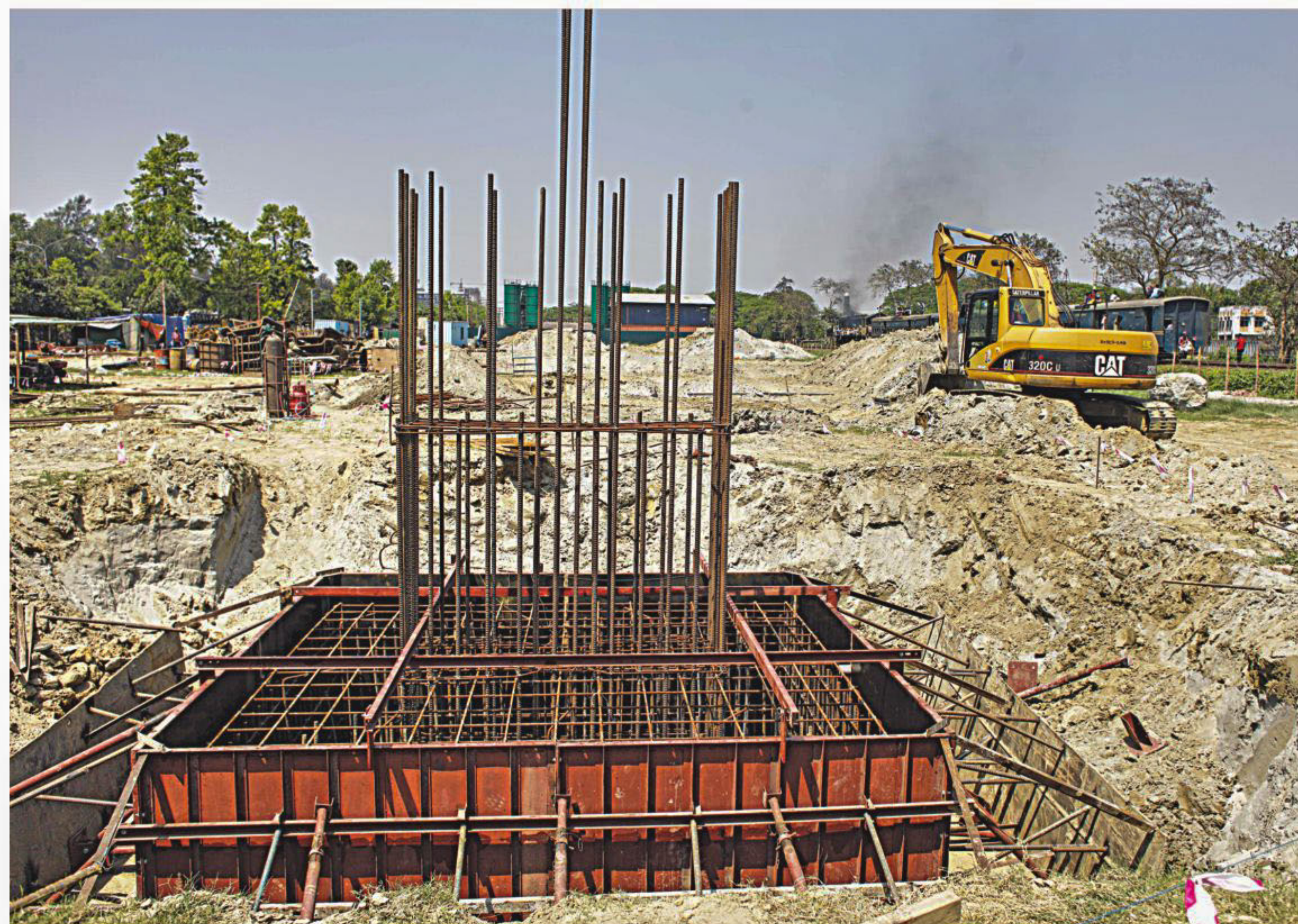
The construction work of the country's first-ever elevated expressway to connect the capital's north with the south started on a limited scale. Once completed, the expressway is expected to ease traffic in the city significantly. The photo was taken in Kaula Railgate area near Airport Railway Station on March 17.
