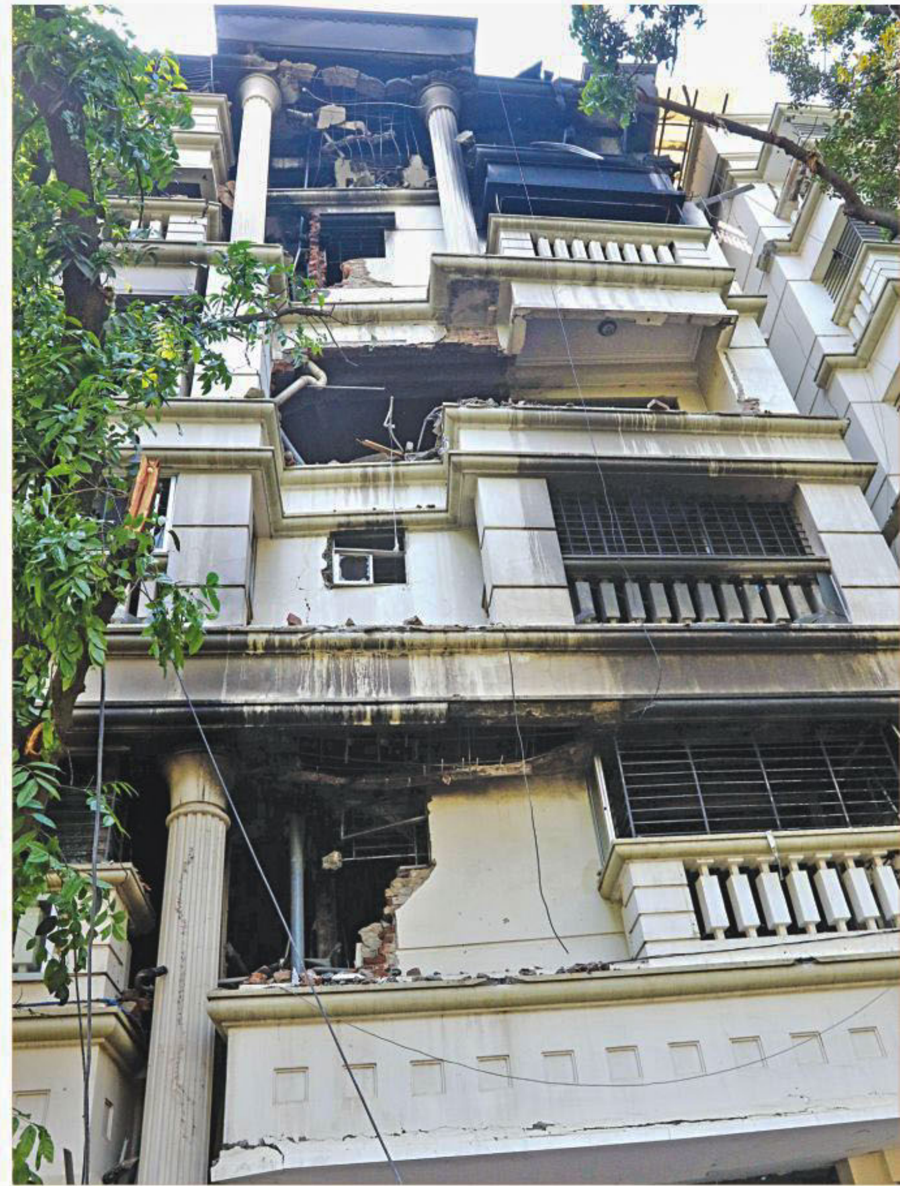
The six-storey building that was badly damaged by a blast in the city's Banani early yesterday. Residents suspect that the blast was caused by a gas leakage.
