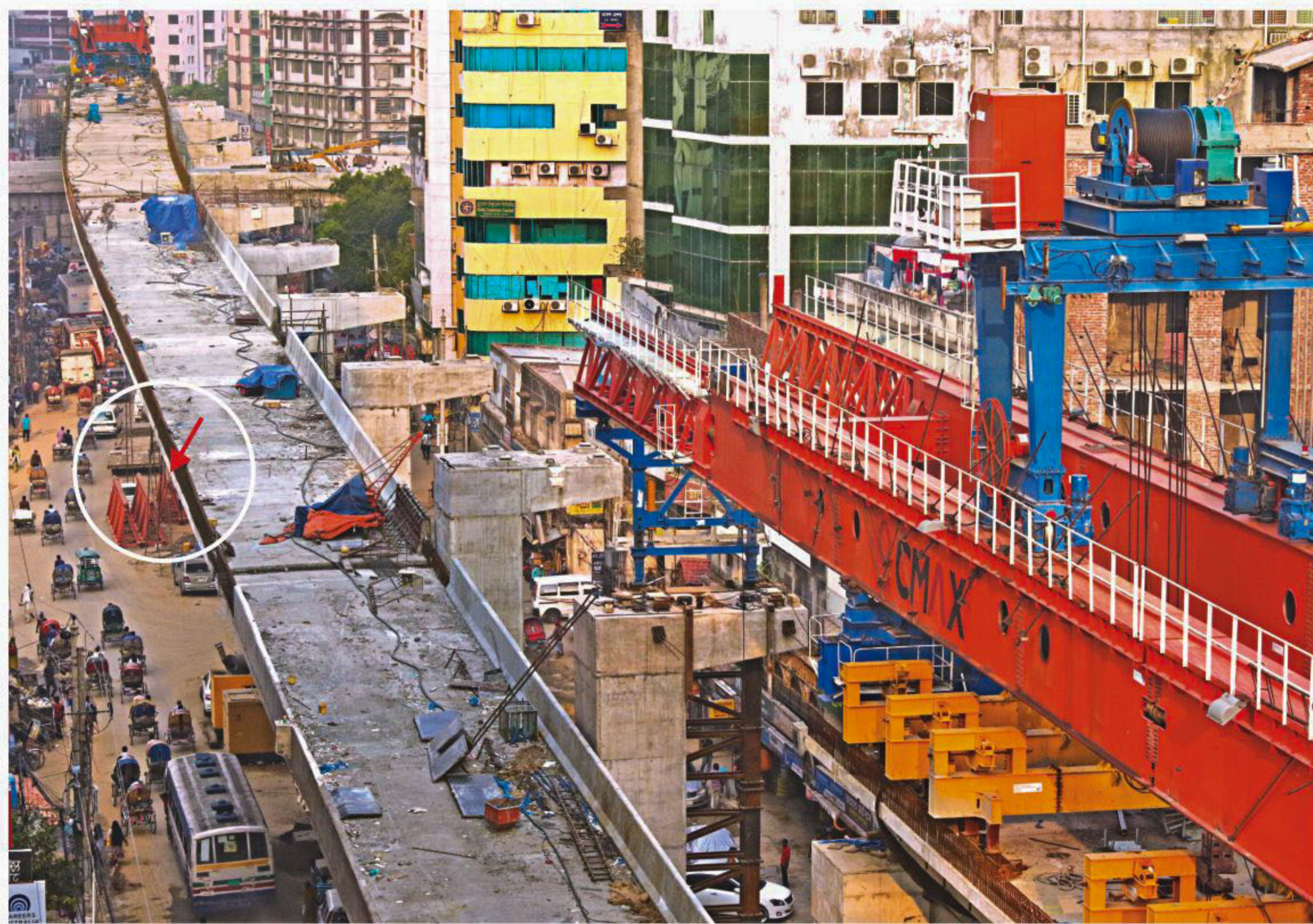
The point, circled, of the under-construction Moghbazar-Malibagh flyover in Eskaton from where an iron bar fell on a worker underneath and killed him yesterday. Construction of the 8.7km flyover in the capital is going on without ensuring adequate safety measures, putting the workers' lives and public safety in peril.
