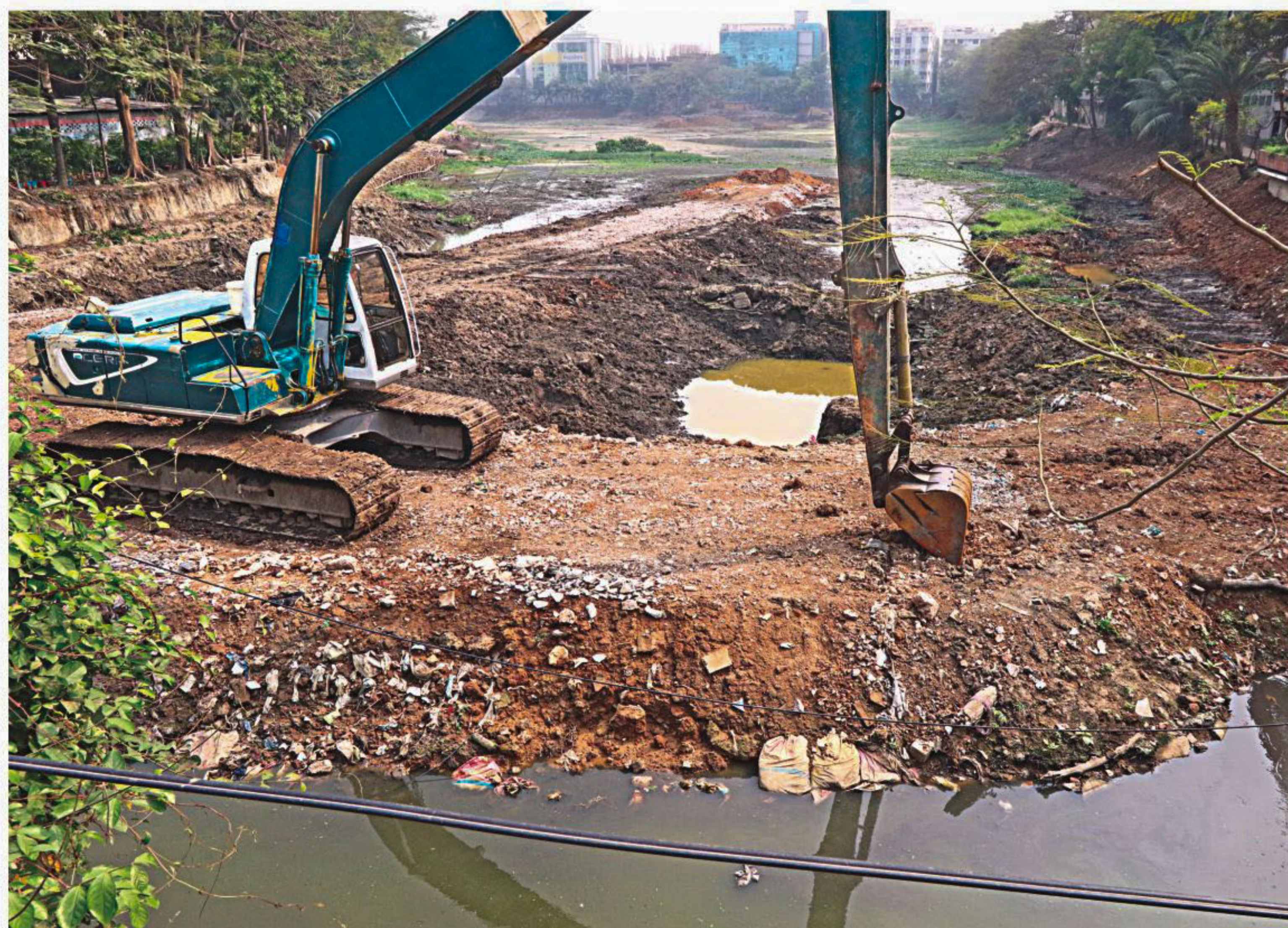
An excavator in operation at Gulshan Lake in the capital's Banani area yesterday. The Rajdhani Unnayan Karttripakkha, the authority to oversee the development of the capital city, has recently taken up a project to restore and augment the beauty of the lake.
