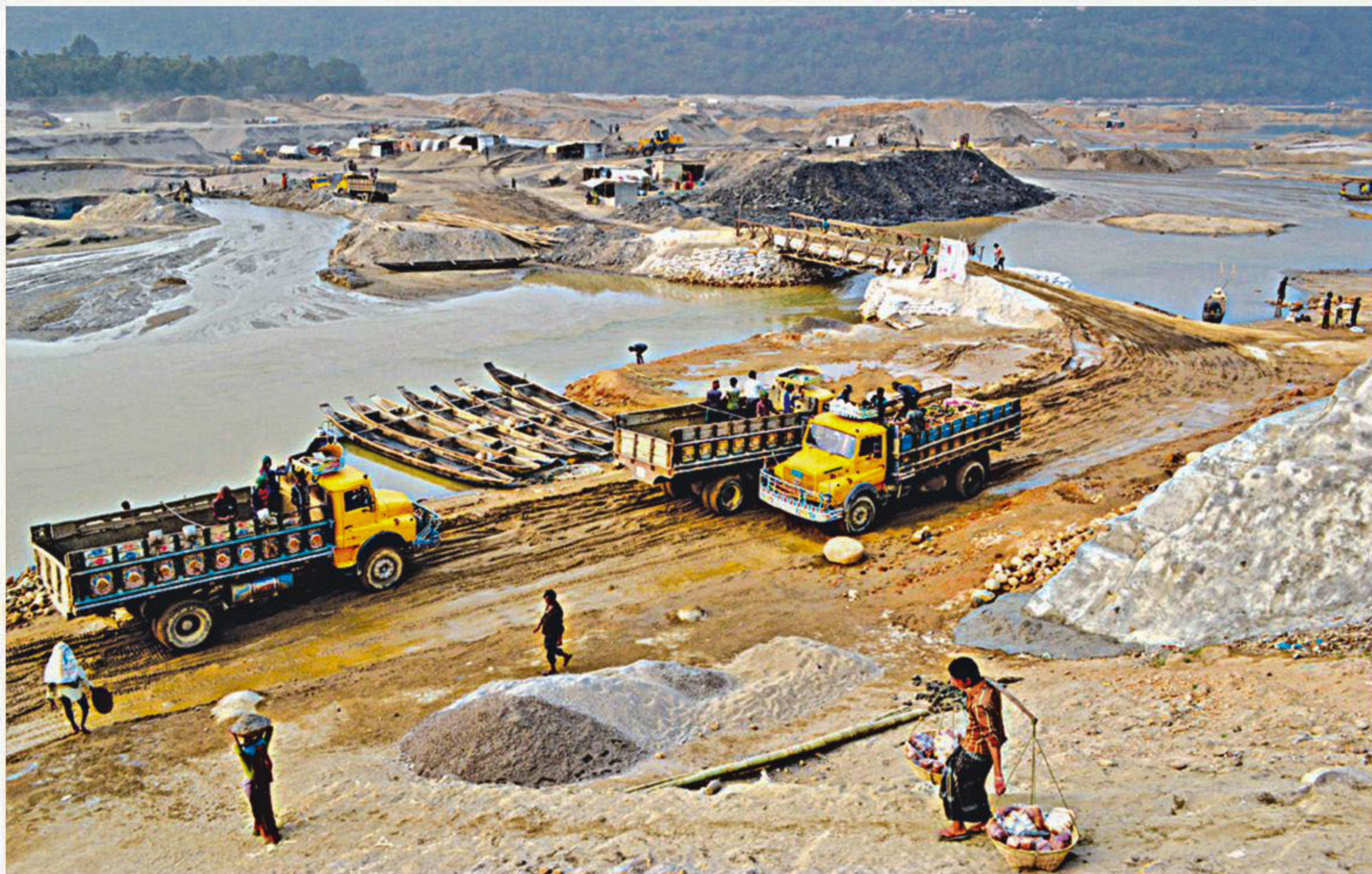
This wooden bridge over the Pyain River in Jaflong of Sylhet has been built illegally by a section of stone traders to facilitate the movement of stone-carrying trucks. It blocks the natural flow of the once pristine river, which has already lost much of its beauty to rampant stone extraction. The photo was taken on Sunday.
