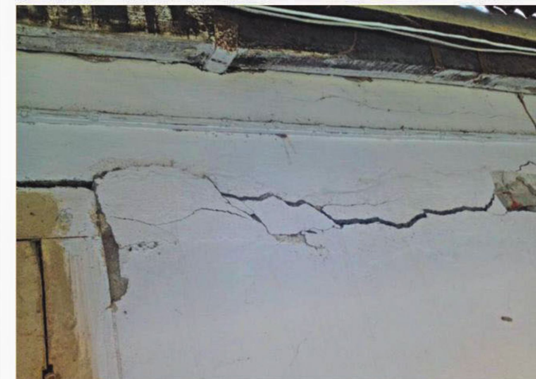
A large crack on a wall of the extension to Al-Biruni Hall of Jahangirnagar University (JU), pictured recently. This one, along with dozens more, was spotted two months ago after the January 4 earthquake, drawing the attention of authorities. However, no step has been taken to repair the hall or evacuate it for the safety of the 200 resident students. Furthermore, first-year students were given allotments at the dormitory.
