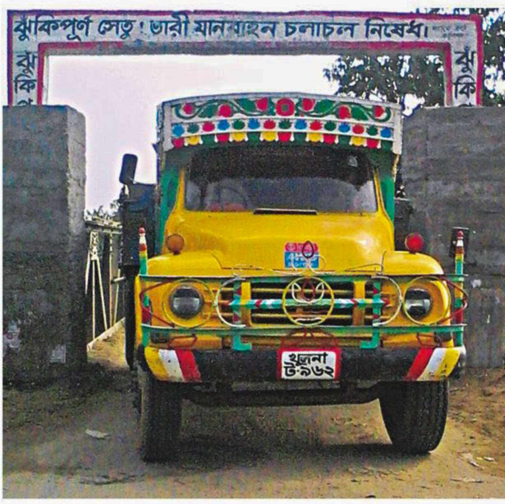
A truck crosses the rickety Bhakurta Steel Bridge over the Turag river even though a large sign on the bridge forbids heavy vehicles from using it. The Daily Star published a similar photo of the bridge at the beginning of this month, mentioning the risks involved. But the authorities have apparently done nothing yet to repair it.
