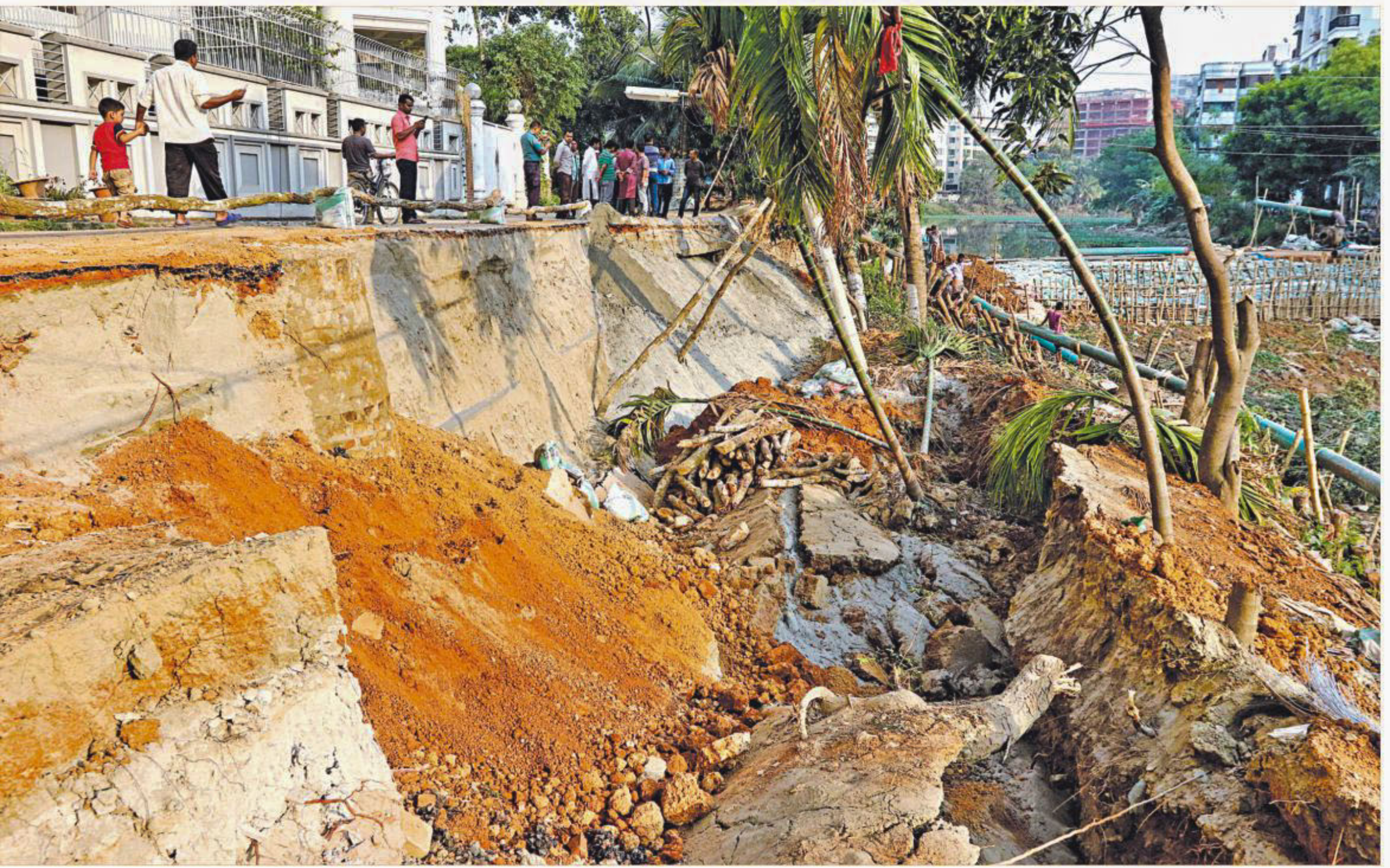
A portion of Road-55 in the city's Gulshan-2 caved into Gulshan Lake yesterday afternoon, putting the buildings on the road in danger. This happened as Rajdhani Unnayan Kartripakkha is implementing a lake beautification project there without ensuring proper safety measures, locals alleged. PHOTO: ANISUR RAHMAN
