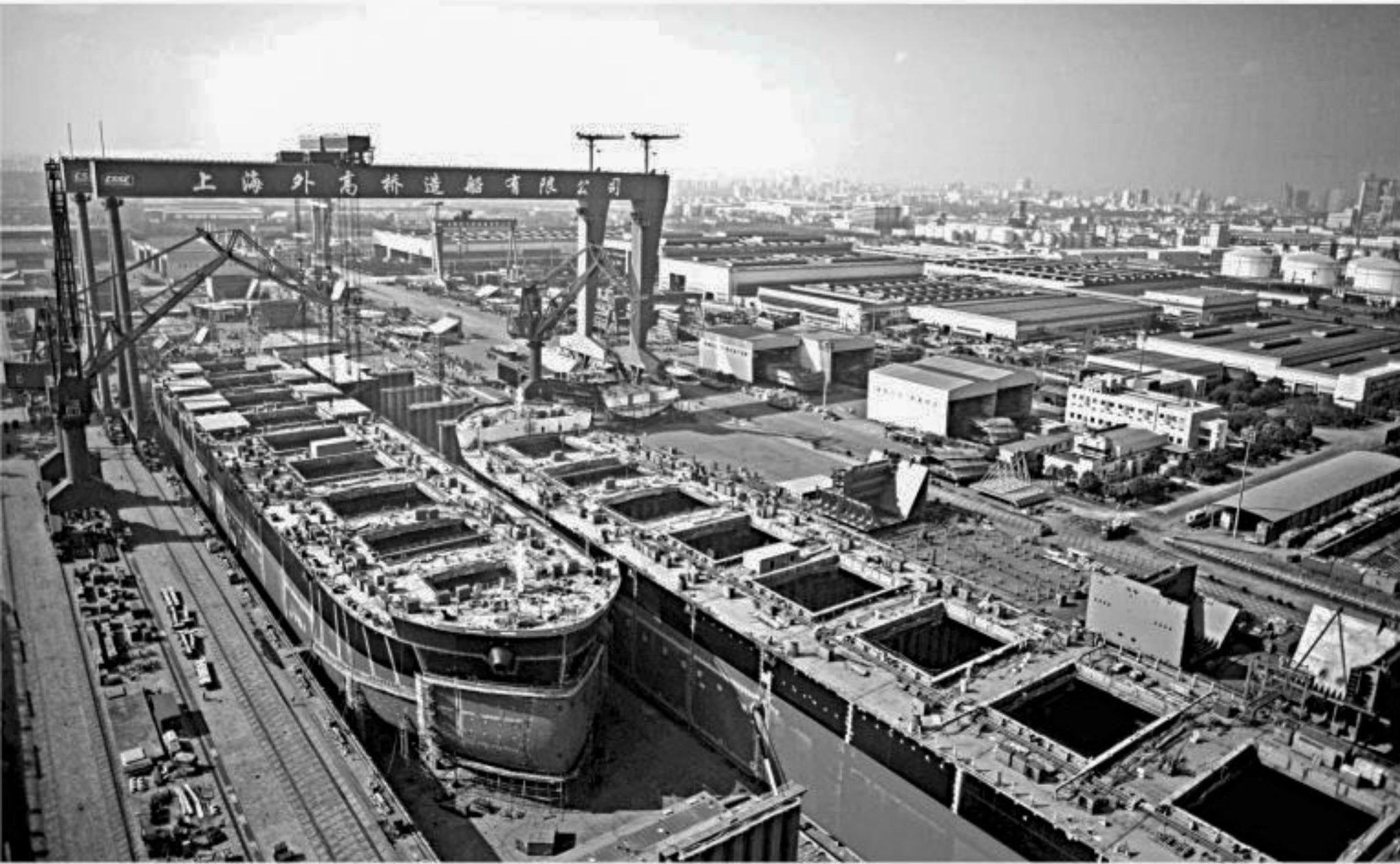
A vessel is seen under construction at the Waigaoqiao shipyard in Shanghai. China's gross domestic product expanded 6.9 percent in 2015 -- its worst performance in a quarter of a century and a far cry from the years of double-digit increases.
