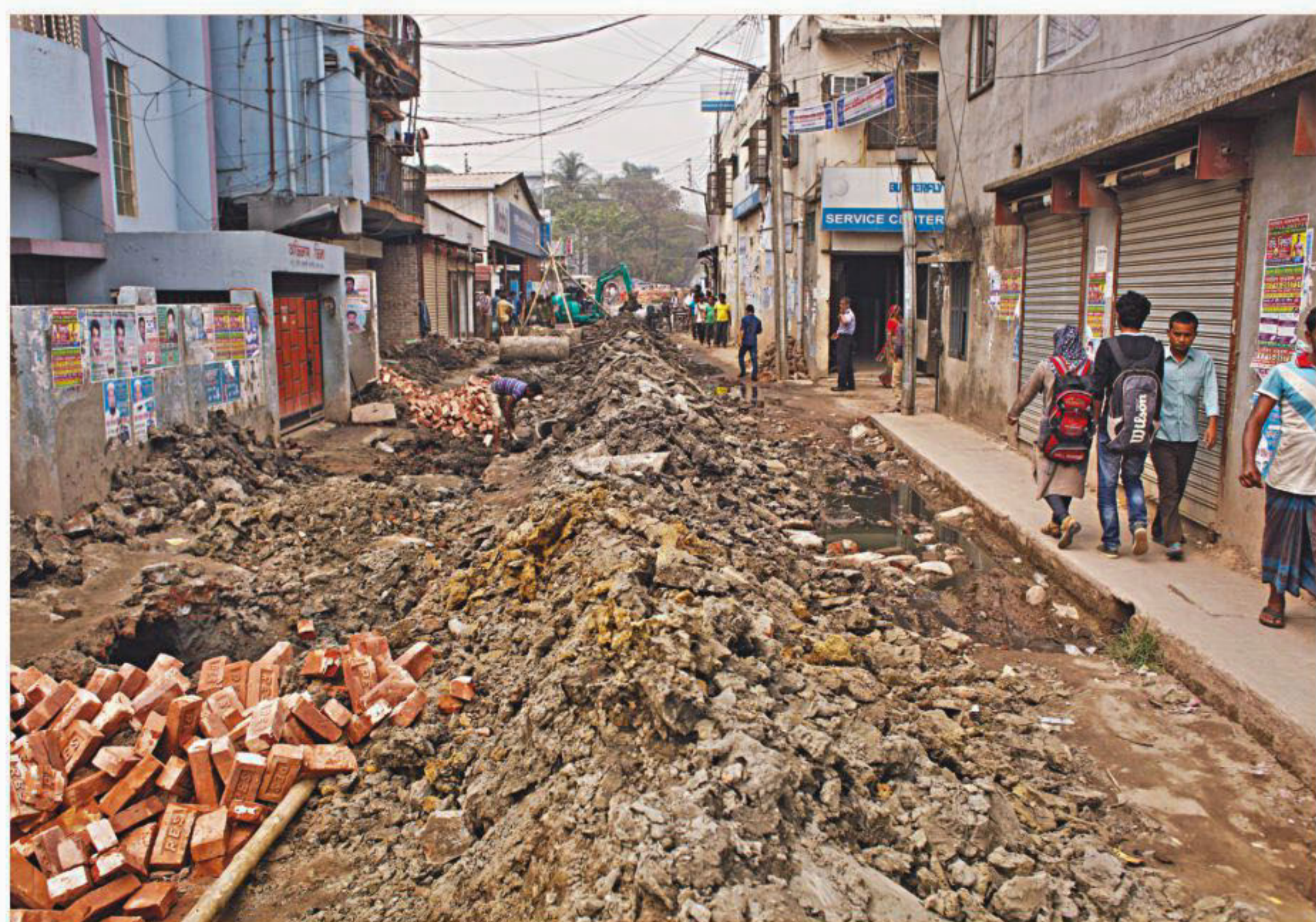
Heaps of earth and construction material are kept on Hatirjheel- Saatrasta Link Road in the capital for quite a few days, completely blocking a footpath and causing huge sufferings to pedestrians.
