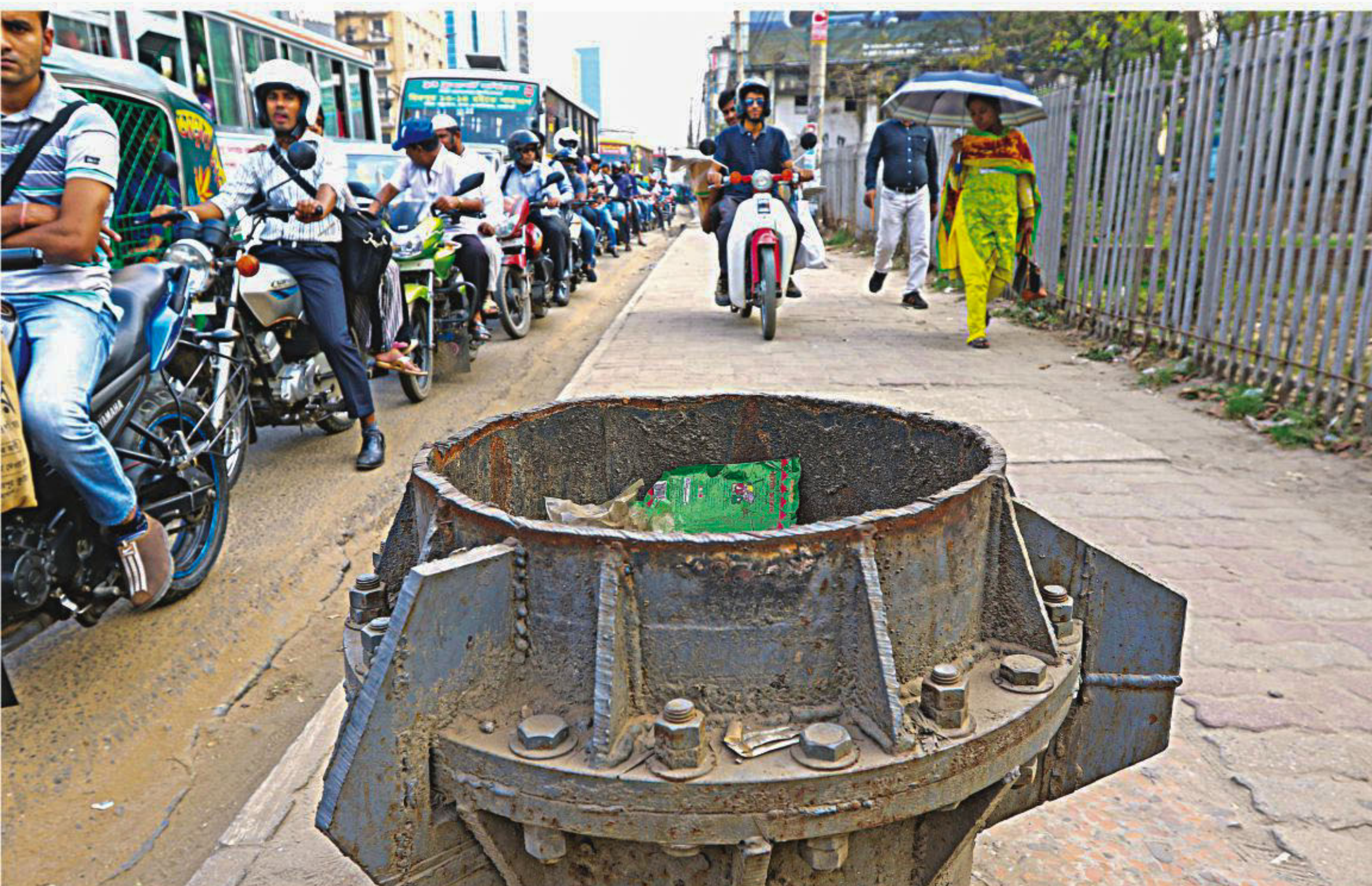
Although the city corporation authorities have removed a billboard right on a pavement of Kazi Nazrul Islam Avenue in the capital, the stump of the billboard's pole remains, causing troubles for pedestrians. The photo was taken in front of Pantha Kunja Park yesterday. PHOTO: PALASH KHAN
