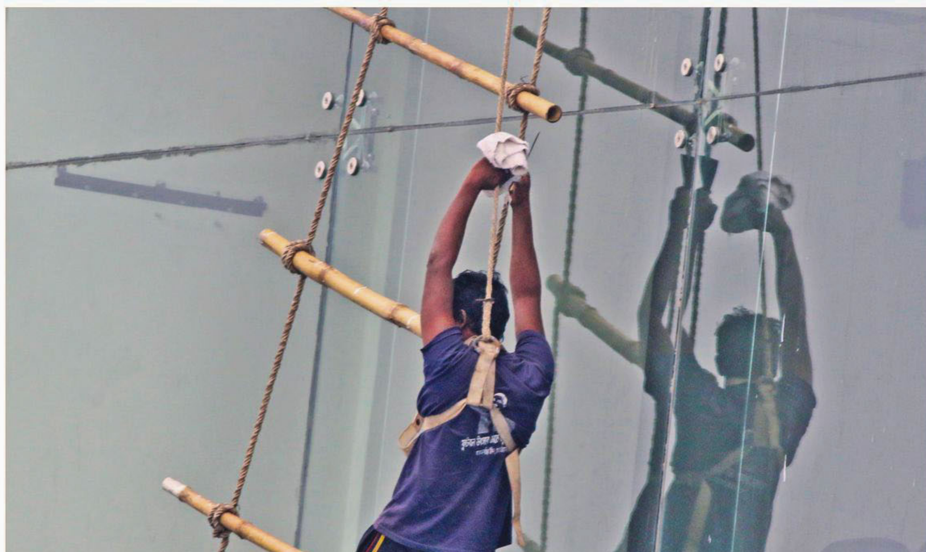
A man on a flimsy rope ladder swaying in the wind trying to gain a balance while cleaning the glass façade of a five-storey building in Sagarika area of Chittagong city yesterday. Though his upper body is tied to a rope by a belt, he has no steady footing. Many of such cleaners usually do not even have that belt either, and often die from losing balance. There needs to be a strict regulation for companies that are in the building cleaning business, and always look to cut corners to maximise their profit at the expense of the lives of cheap labourers.
