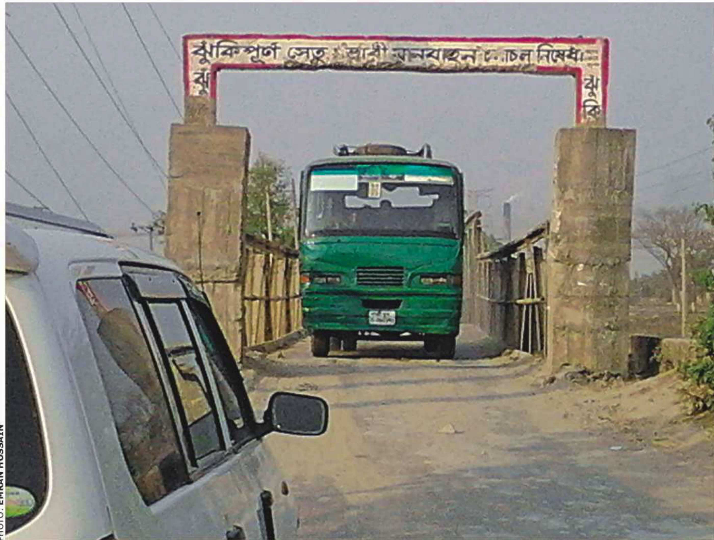
A bus crosses the squeaking and rattling Bhakurta Steel Bridge over the Turag yesterday even though a large sign on it forbids heavy vehicles from using the bridge. Even trucks use the bridge every day. Contacted, authorities concerned could not say anything about the condition of the bridge or who put the sign there. About 30,000 residents of 27 villages in Bhakurta union of Savar use the bridge.
