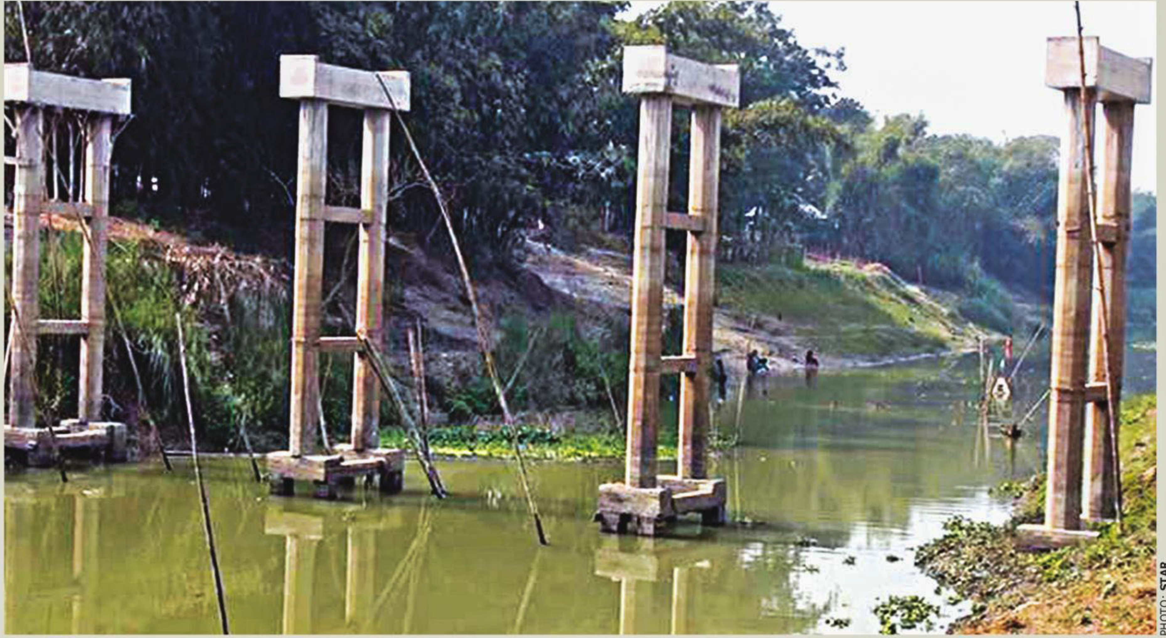
An under-construction bridge over a canal at Palora Mollar Ghat in Manikganj -- an initiative of people from seven villages. The photo was taken early this month.
