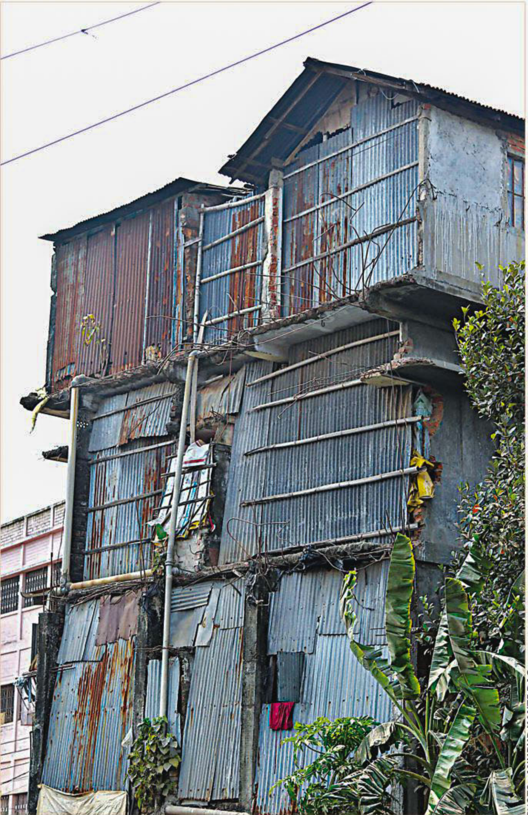
This weird-looking structure is actually a residential building at Mia Khan Nagar of Chittagang city. It's hard to imagine how the building, partly made of concrete and partly of corrugated iron sheets, is still standing. Even a mild earthquake or a landslide may cause a major accident there. The photo was taken yesterday.
