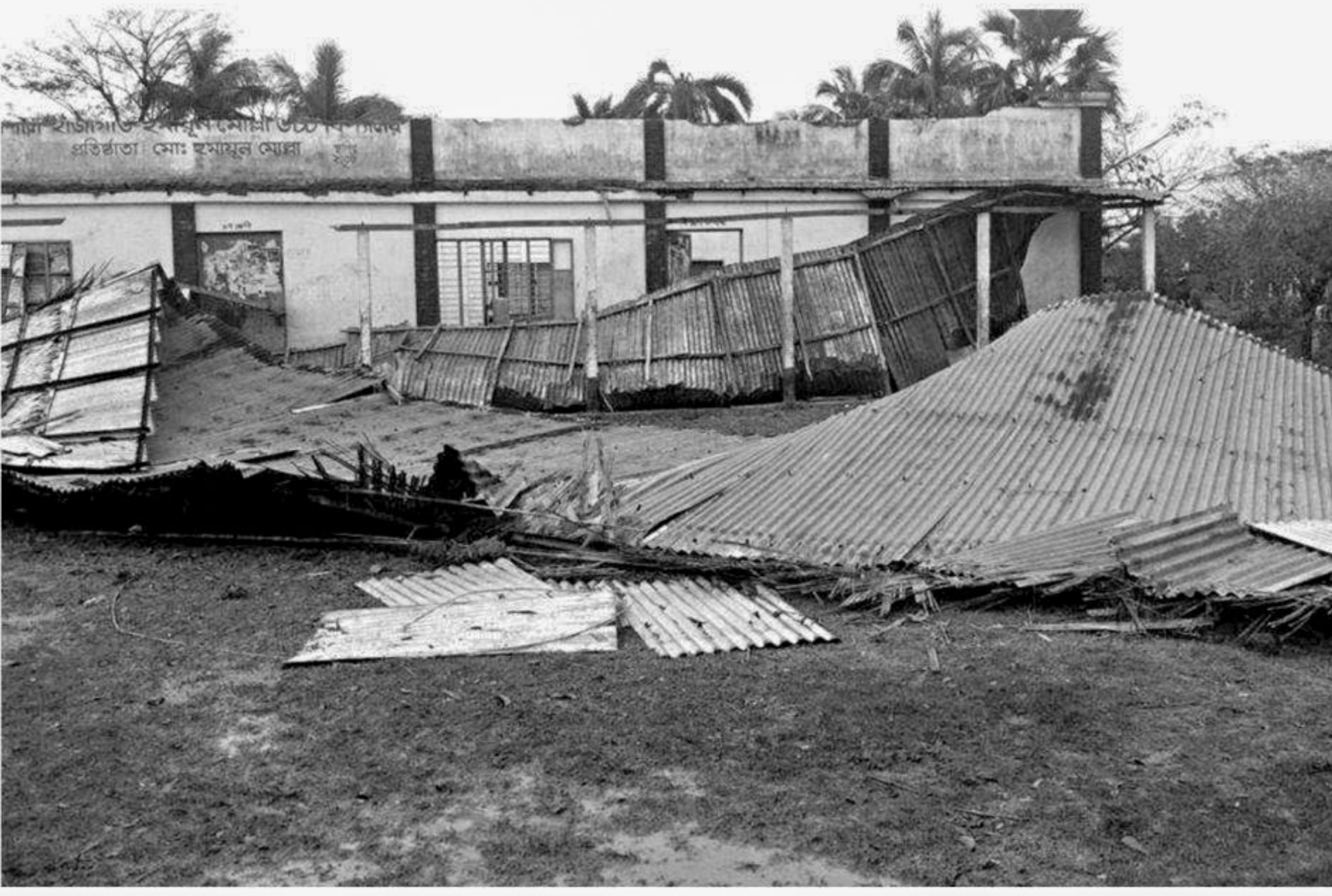
A storm blew off the tin-roof of Humayun Molla High School in Sirajdikhan upazila under Munshiganj district yesterday.
