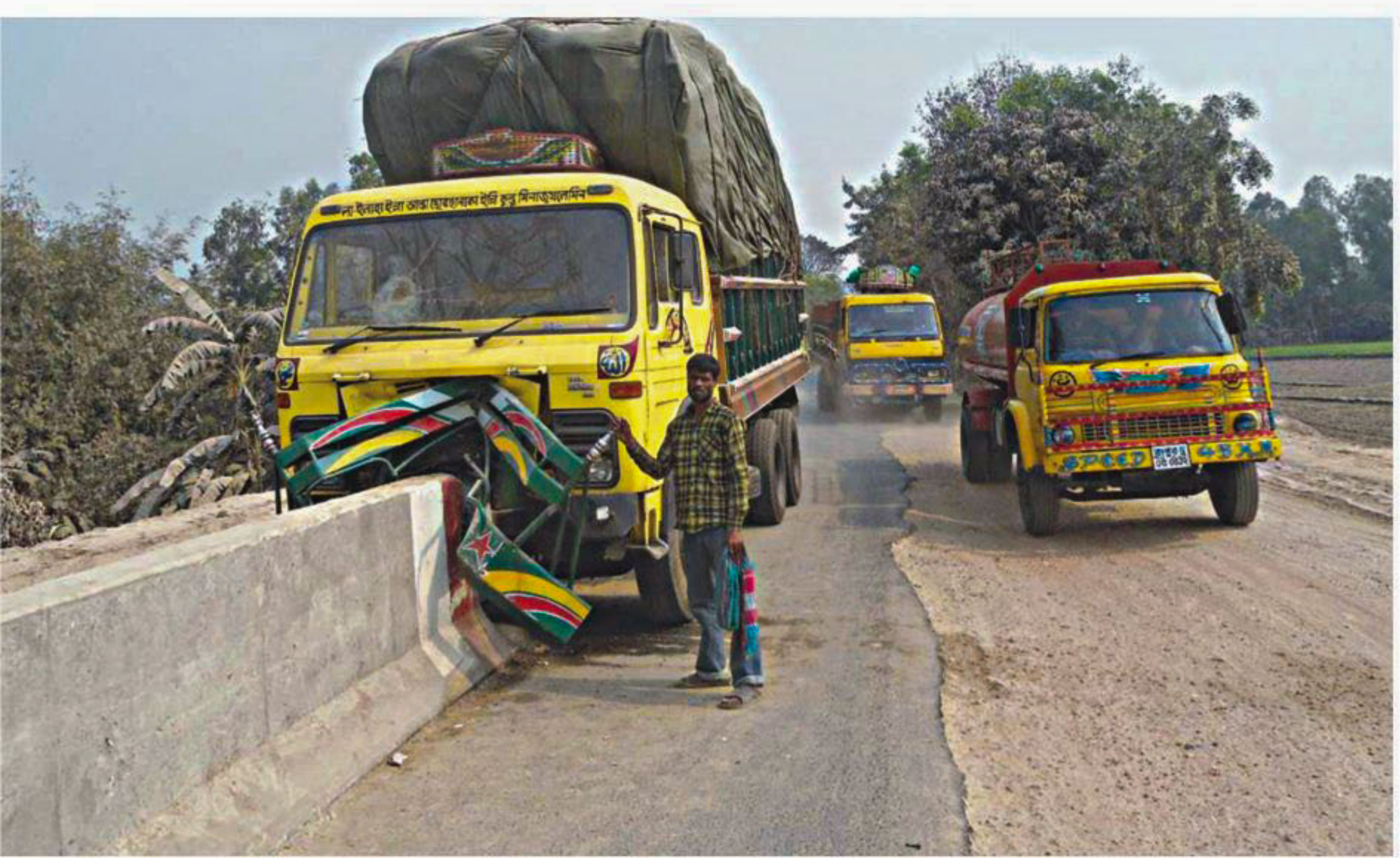
A truck hit this incomplete road divider on Panchagarh-Dinajpur highway at Untrish Mile village in Thakurgaon Sadar upazila a few days ago. Such accidents have become frequent as the work for setting up road divider and expansion of the road has remained incomplete for around six months, leaving several spots of the road highly risky for vehicles.
