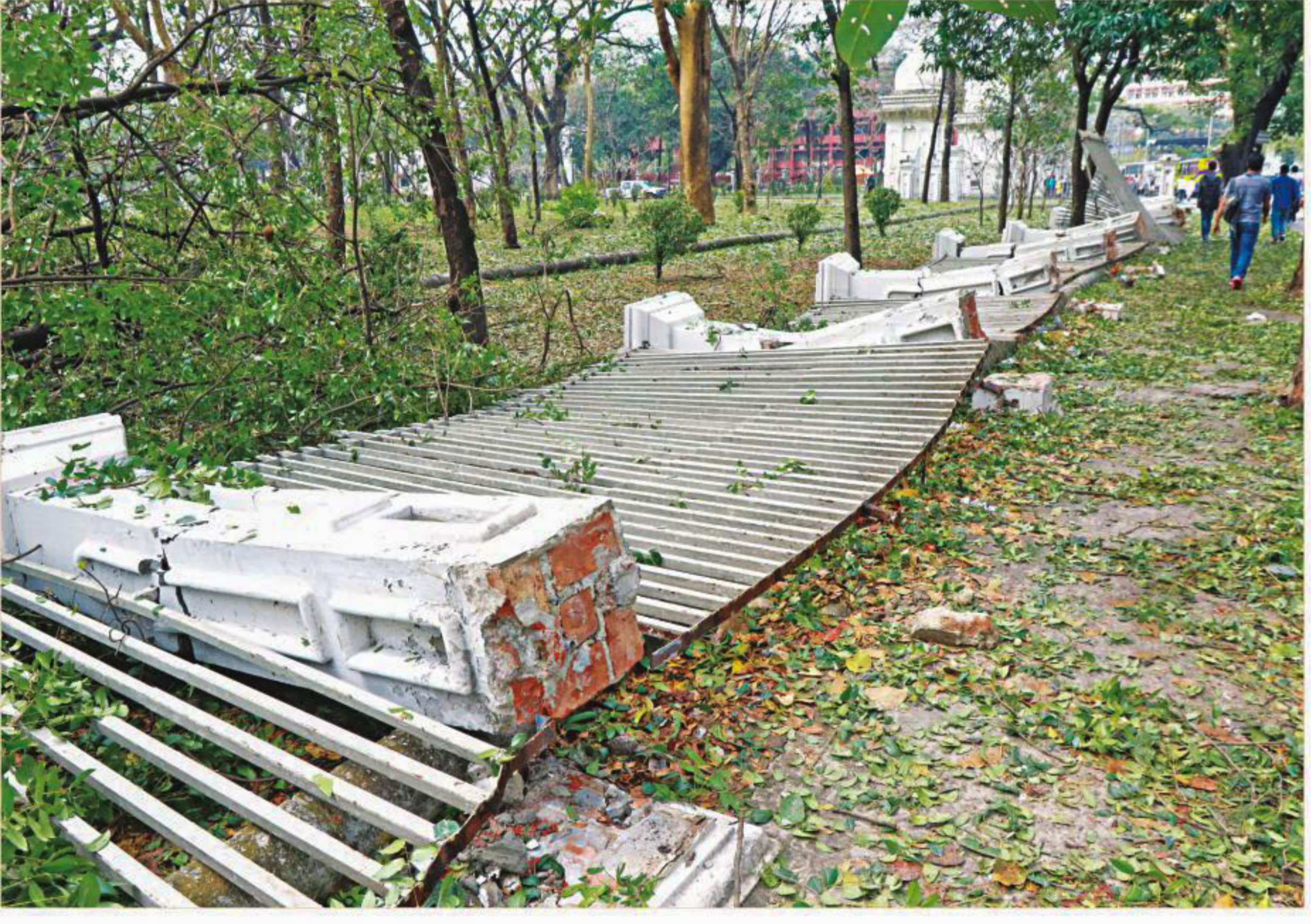
A portion of the Supreme Court boundary wall that collapsed during a midday hailstorm yesterday. Strong winds also uprooted a tree there.
