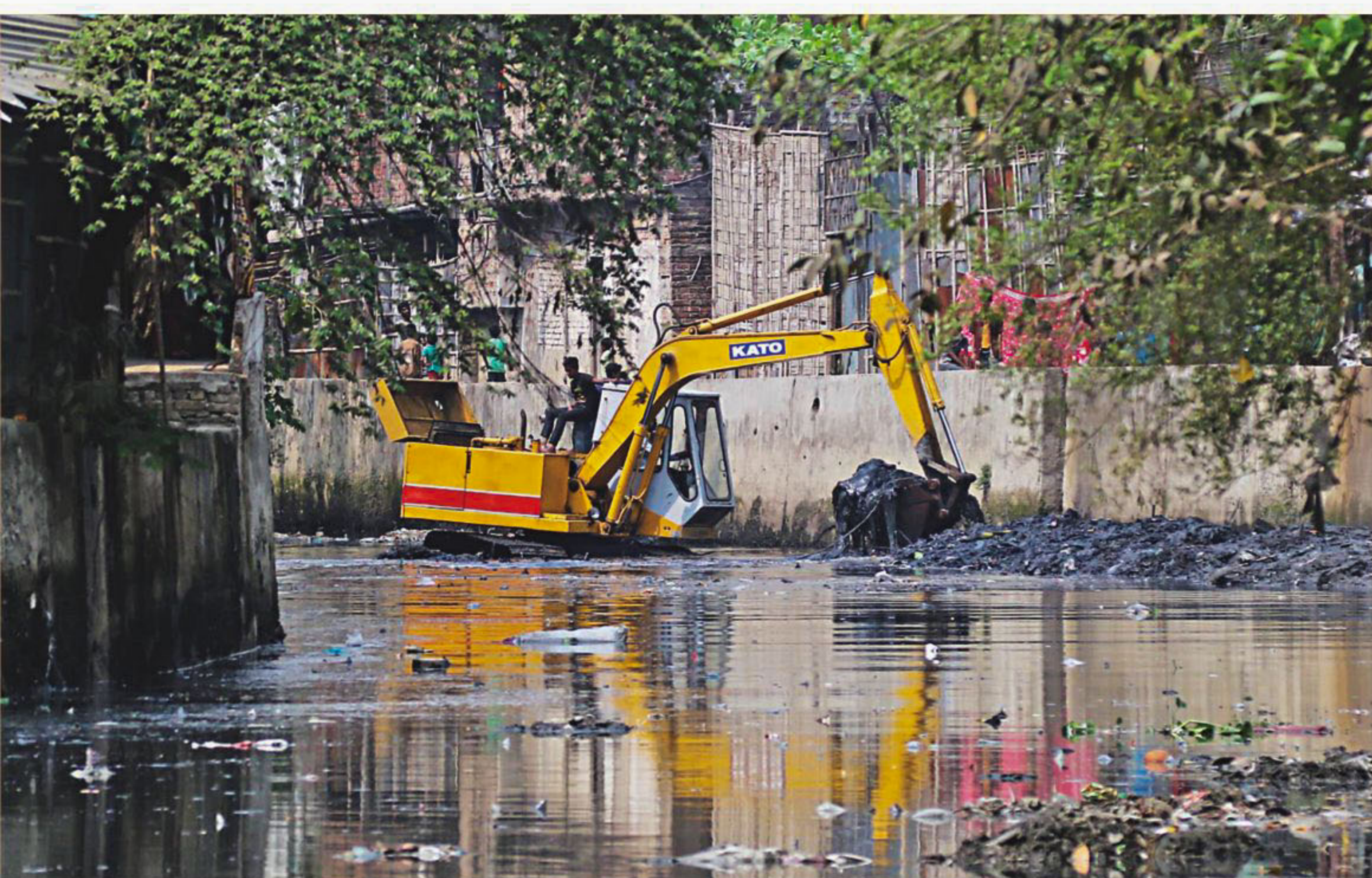
Re-excavation and cleaning of Chaktai Khal going on in Chittagong city yesterday. Following reports published by different media, including The Daily Star, the city corporation finally started the drive on the canal early this month to avert waterlogging during the upcoming monsoon. The authorities want to implement the project within two months. The photo was taken at Bakalia-Bou Bazaar.
