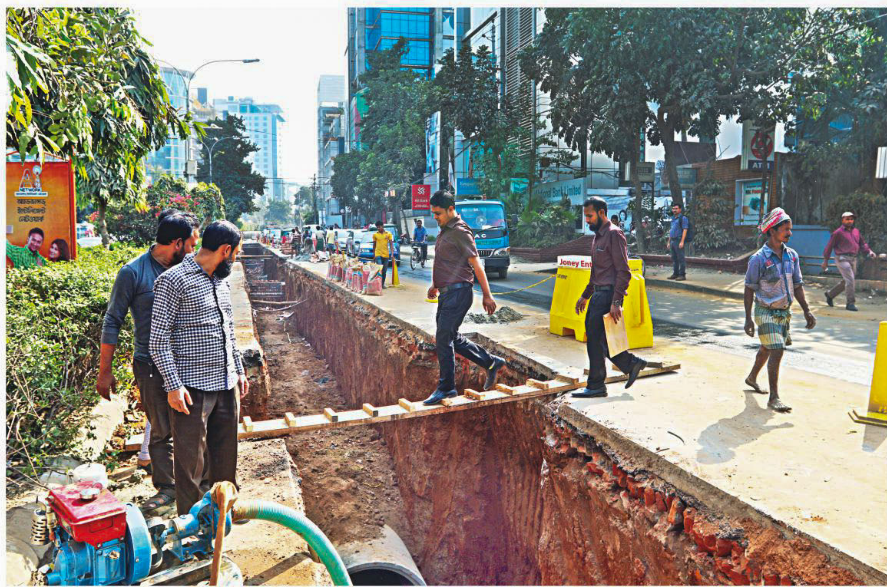
Pedestrians risk their lives using a wobbly plank to cross a dug up section of a road in Gulshan 2 in the capital with Dhaka North City Corporation apparently turning a blind eye to the matter, including properly cordoning off the under construction sites, while installing sewer pipes. The photo was taken yesterday.
