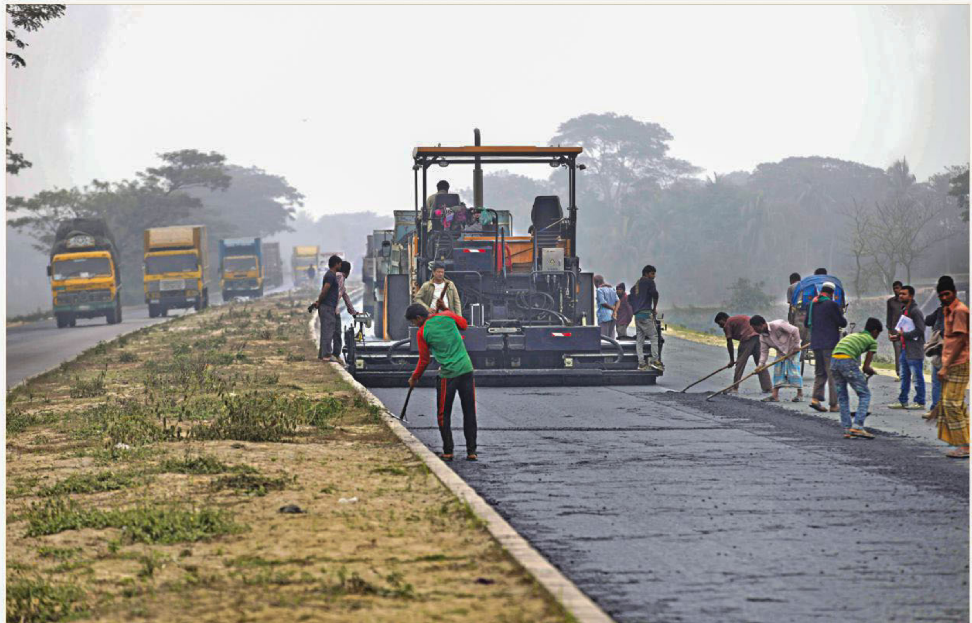
Workers giving a final touch to one side of the dual carriageway in Daudkandi area of Comilla. The photo was taken recently.
