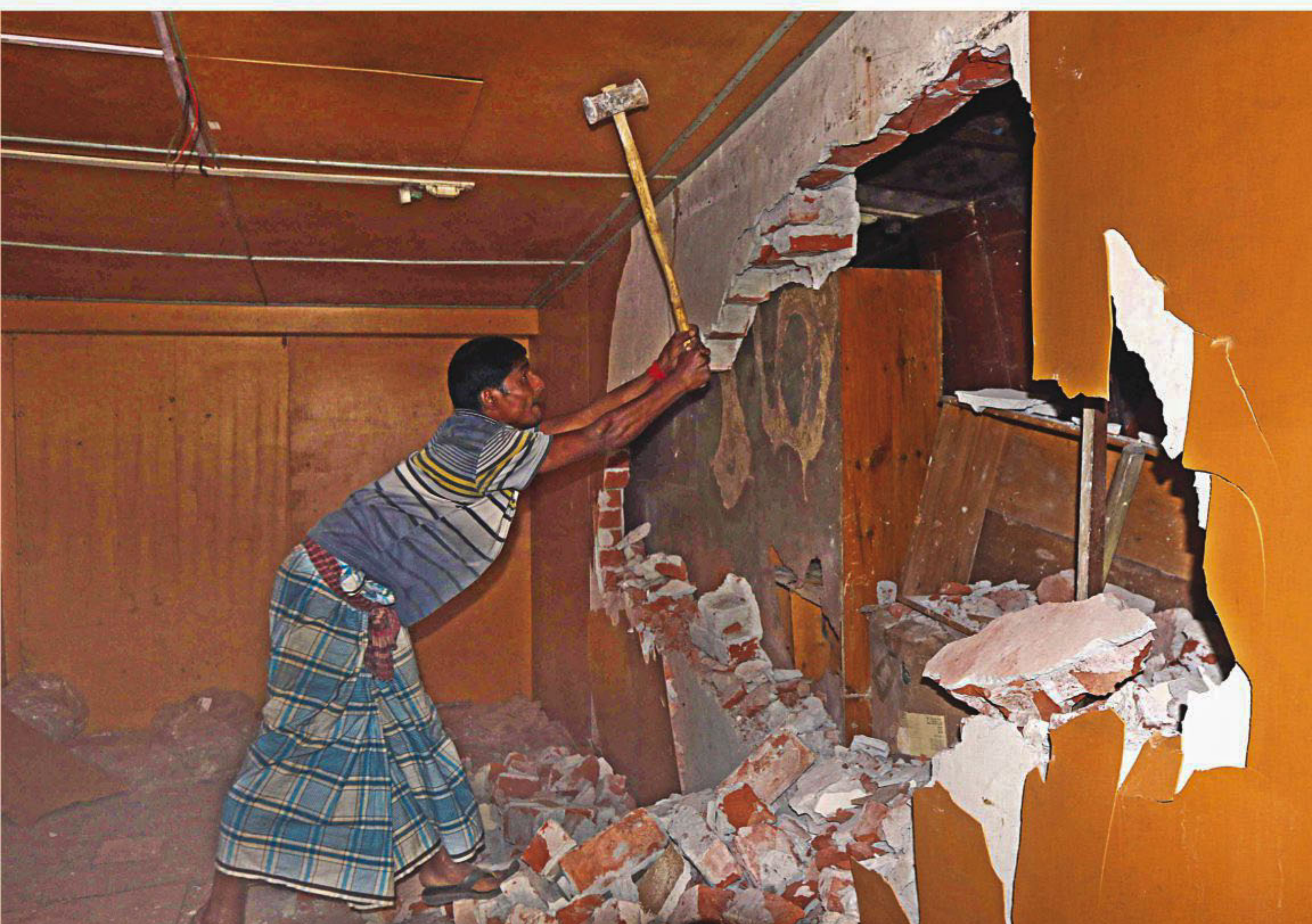
A worker of Rajdhani Unnayan Karttripakkha (Rajuk) knocking down the wall of a building in the city's Mirpur Road during an eviction drive by a Rajuk mobile court yesterday. The house-owner built a warehouse at the designated car park.
