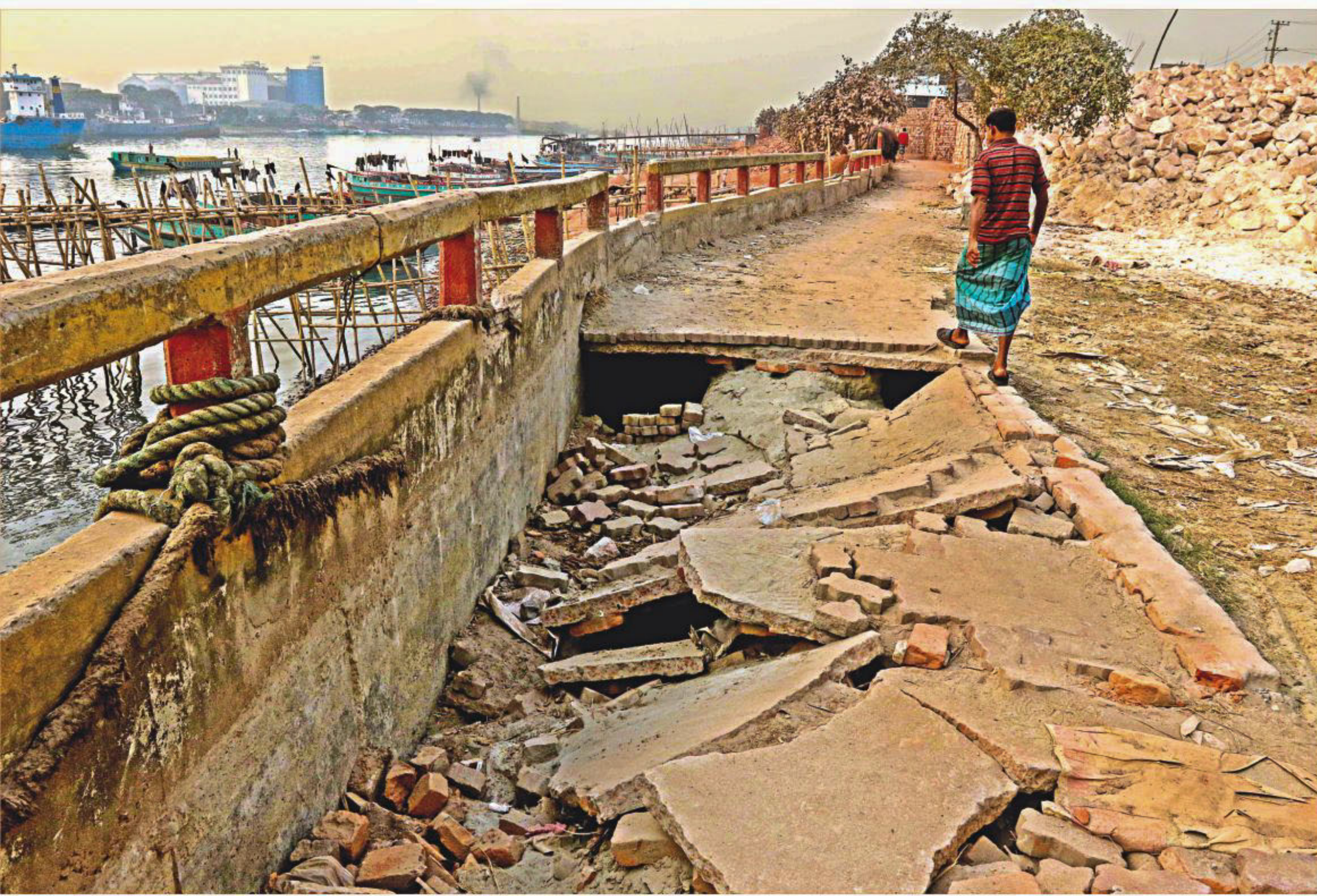
Hard to believe this walkway along the Buriganga river in Pagla of Narayanganj was built only two years ago. Locals claim that poor quality construction material was the reason for the collapse of the pavement. The government built the walkway to keep the river free from occupiers and pollution. The photo was taken recently.
