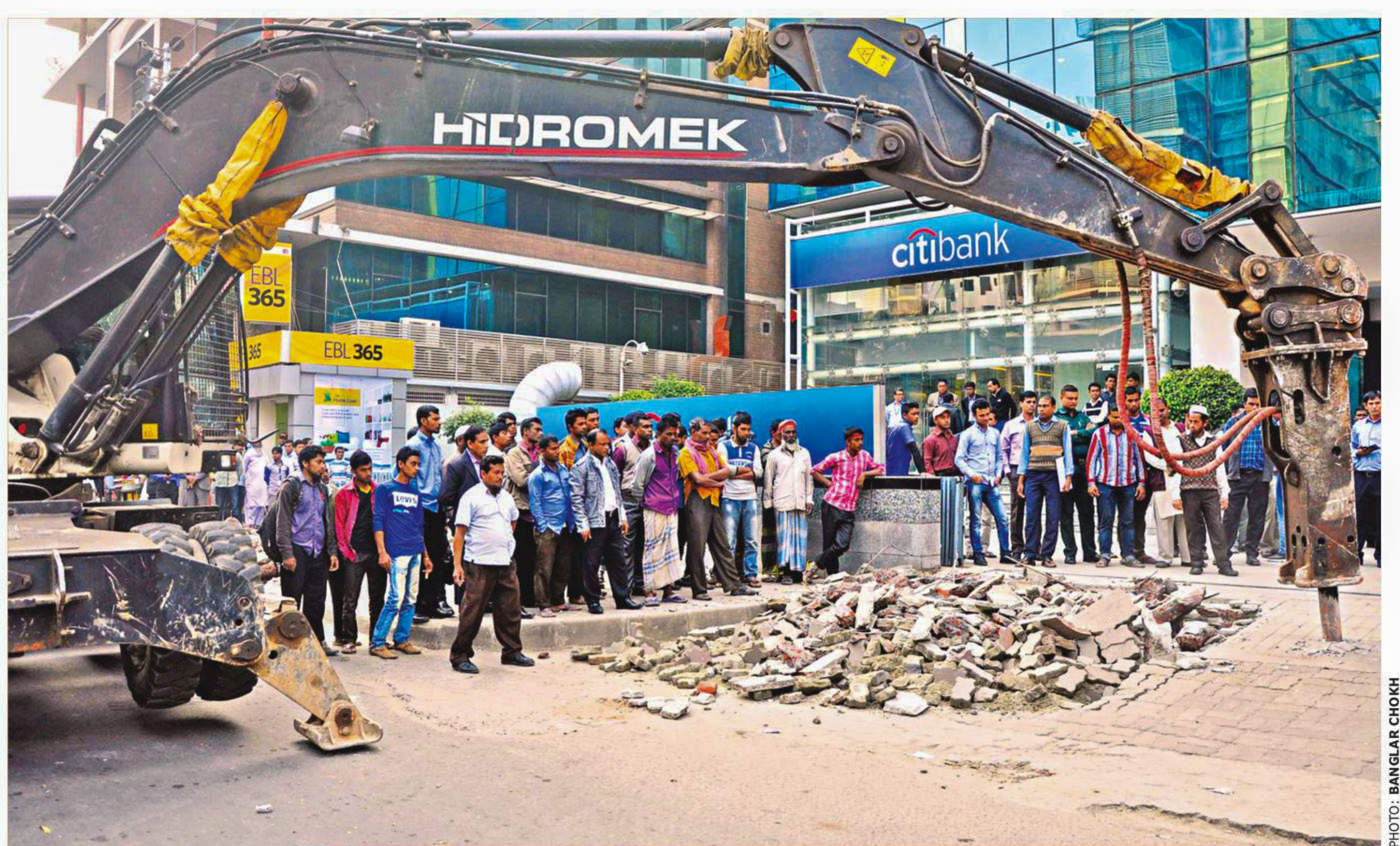
The Rajdhani Unnayan Kartripakkha (Rajuk) dismantling an access ramp built illegally in front of the Citibank office on the capital's Gulshan Avenue yesterday. It was part of the government organisation's continued drives to free footpaths and recover basement car parks from illegal occupation in Uttara, Gulshan and Dhanmondi.
