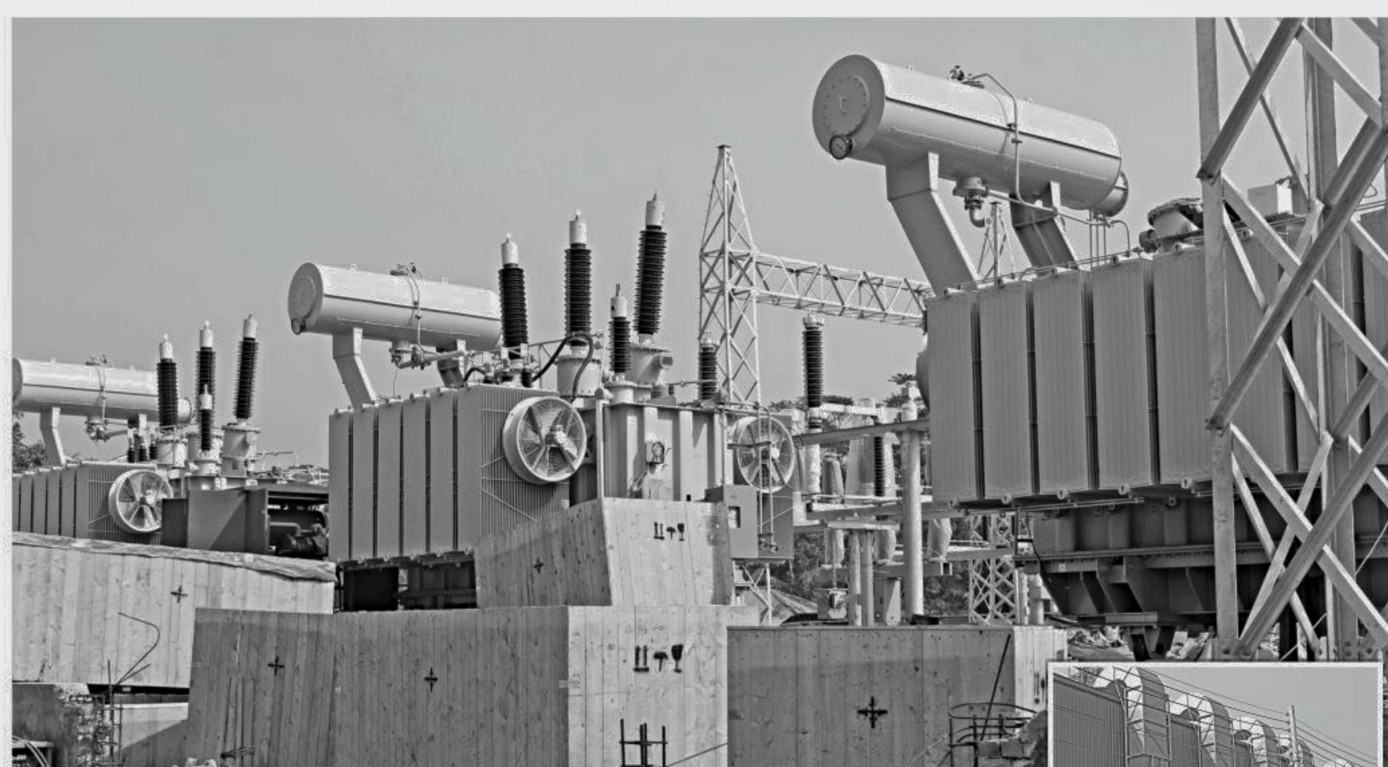
View of the under-construction power plant of Summit Group in Barisal. The plant, set to begin operations in February, will add 112 megawatts of electricity to the national grid.
