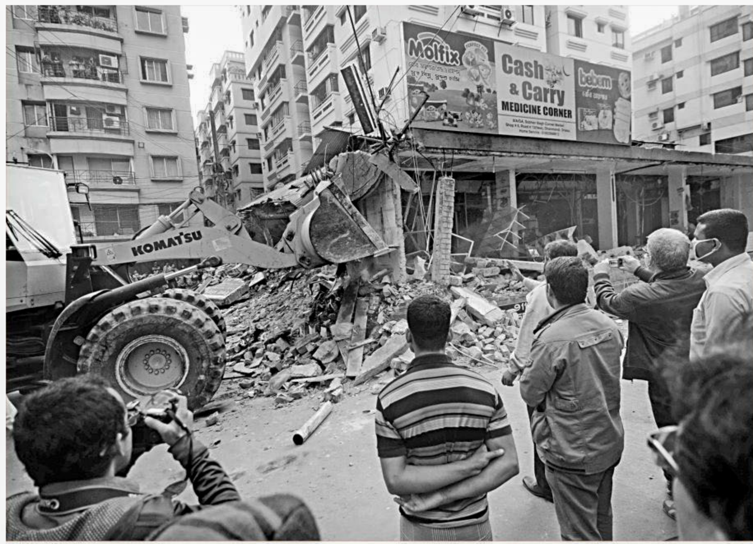
A bulldozer demolishes an illegal structure in the capital's Sobhanbagh yesterday during an eviction drive conducted by a mobile court of Rajdhani Unnayan Karttripakkha.
