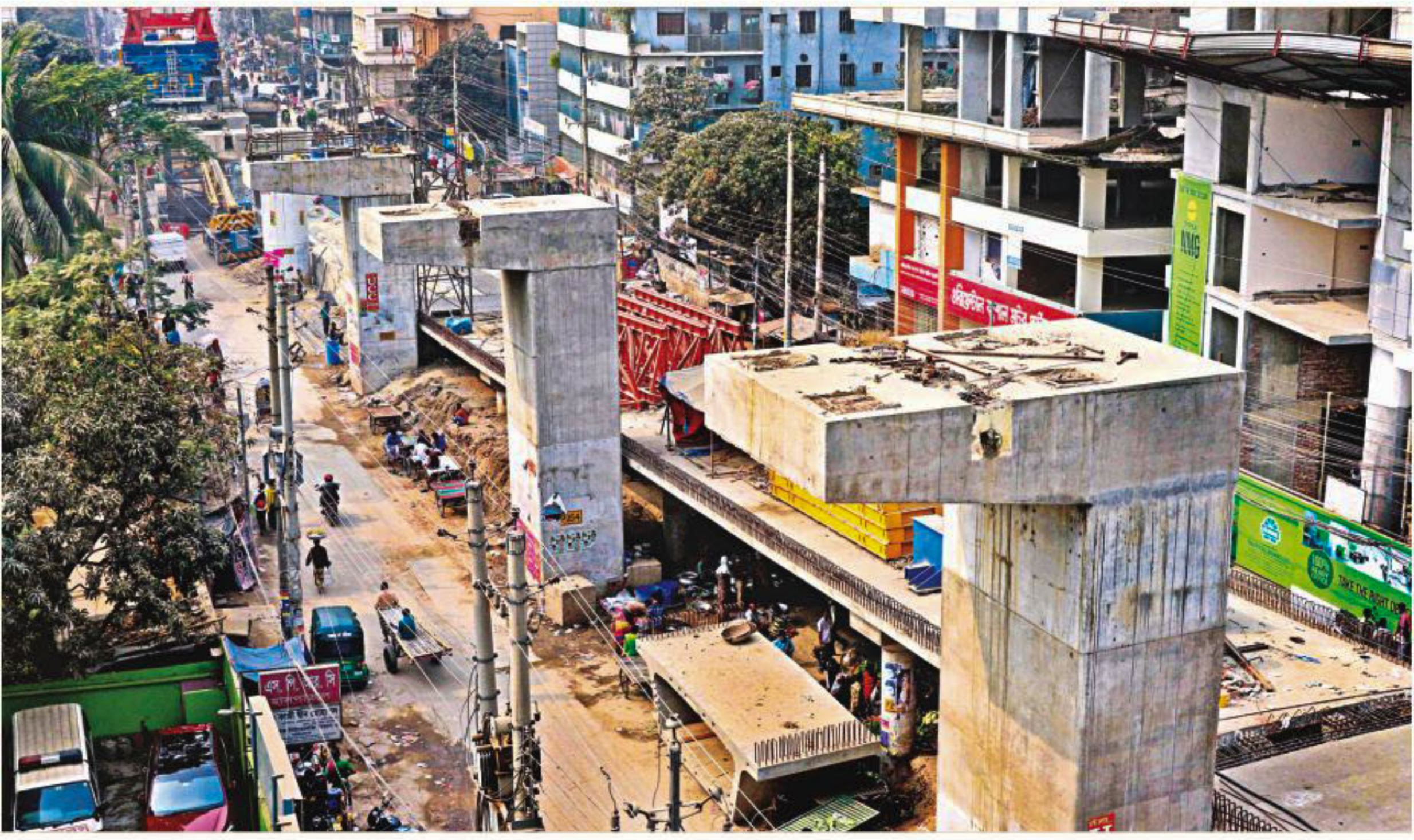
LONGER IN TIME, COSTLIER TO BUILD: The Moghbazar-Mouchak Flyover will take one and half years more to complete and cost more now. The Executive Committee of the National Economic Council yesterday hiked the project cost by Tk 446 crore. The new finishing time is June 2017 from December 2015. Commuters will continue to endure the perennial gridlock in the area. The photo was taken in the city's New Eskaton Road yesterday. PHOTO: AMRAN HOSSAIN
