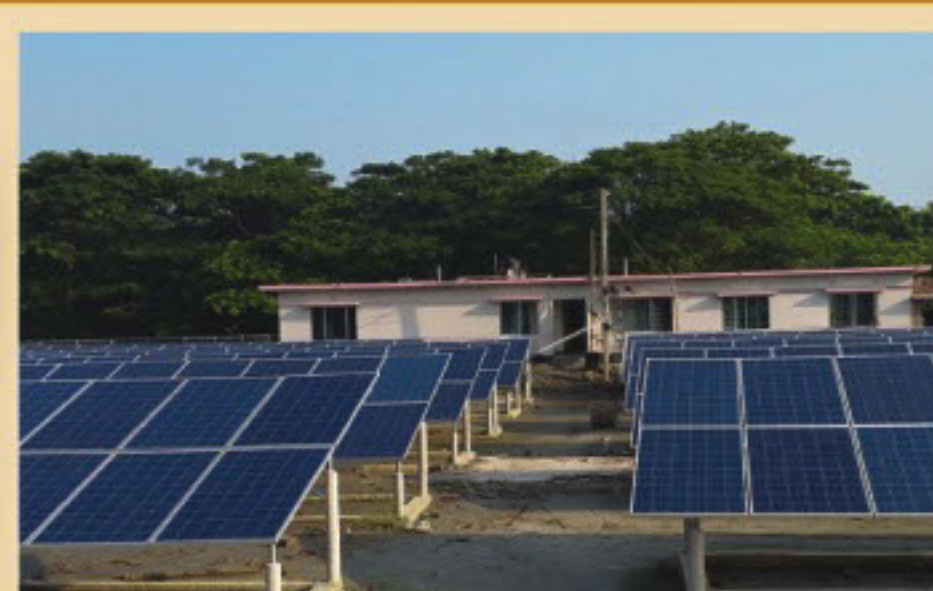
SEBL 177 kWp project at Monpura, Bhola
