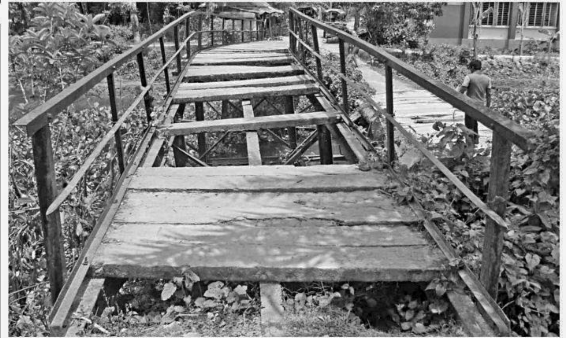
The iron bridge on Humoibunia canal in Amragachhia union of Mirzaganj upazila under Patuakhali district remains in an awful condition for years, disturbing communications on Fakir Haat-Amragachhia road.
