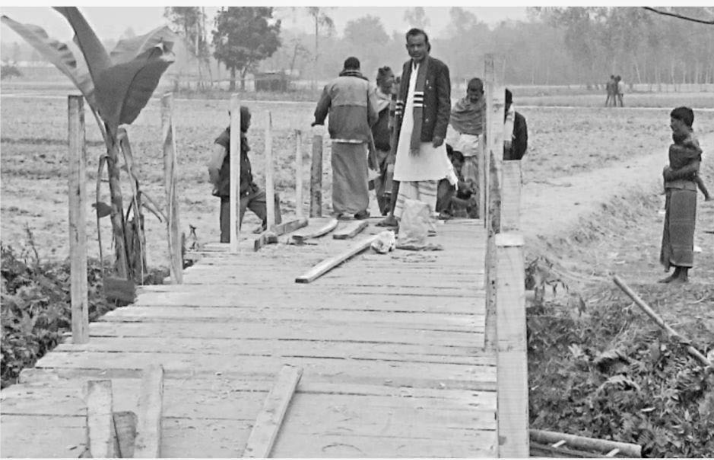
Built with voluntary service of the locals, the wooden bridge at Hajipur village in Nogda Shimul union of Gopalpur upazila under Tangail district gets ready for use on Monday.
