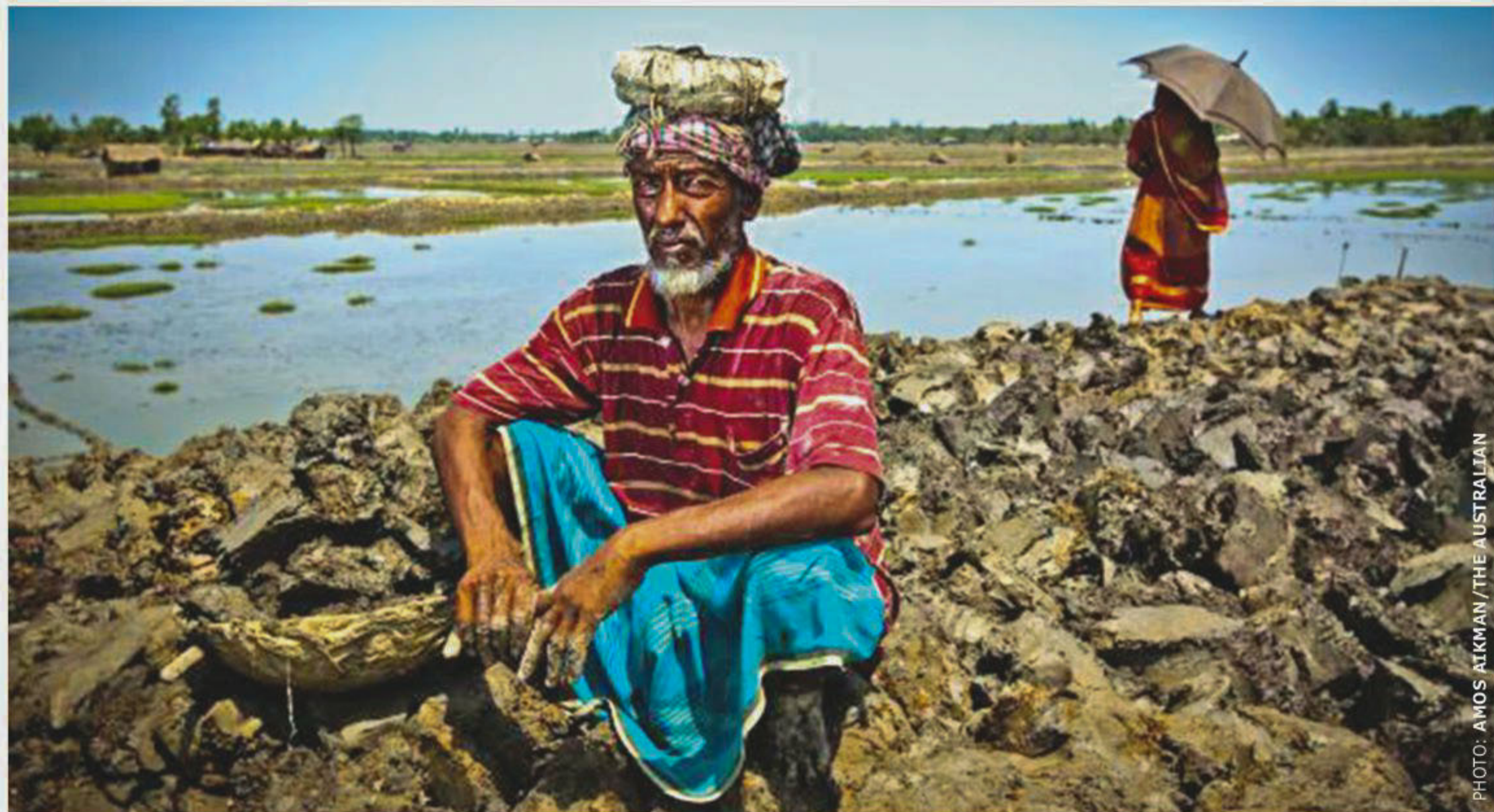
Mohamed Abdul Wozad repairs an embankment protecting Gabura island in south-west Bangladesh from flooding.
