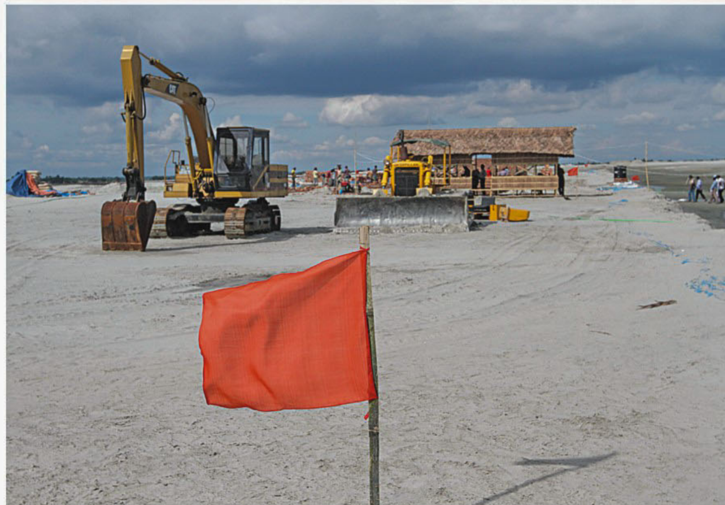
Despite opposition by activists and environmentalists to the Rampal project, construction of the power plant continues unhindered.
