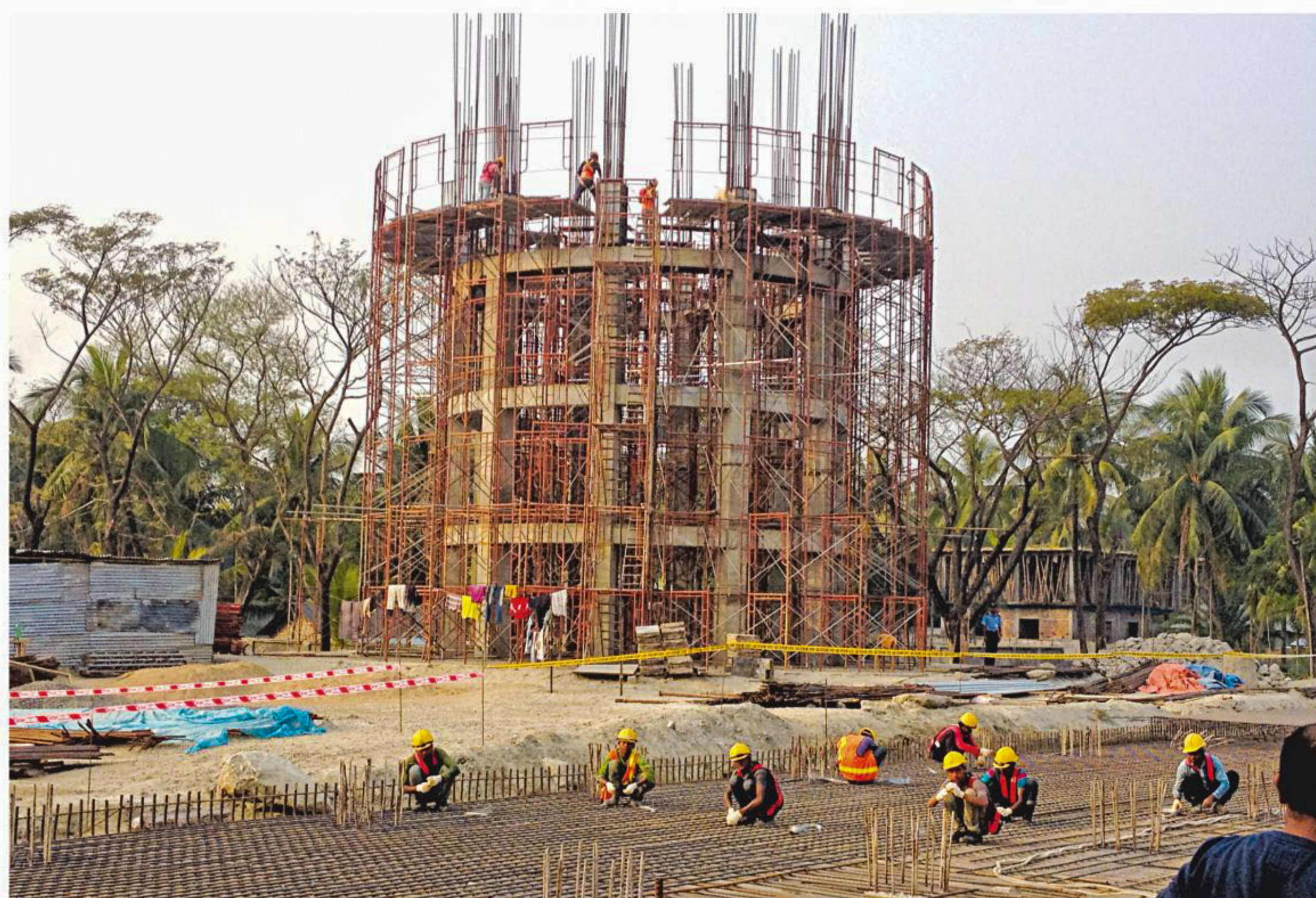
People working at the construction site of a water treatment plant in Khulna. Once in operation, the plant is expected to considerably alleviate the perennial water crises city dwellers face every day.
