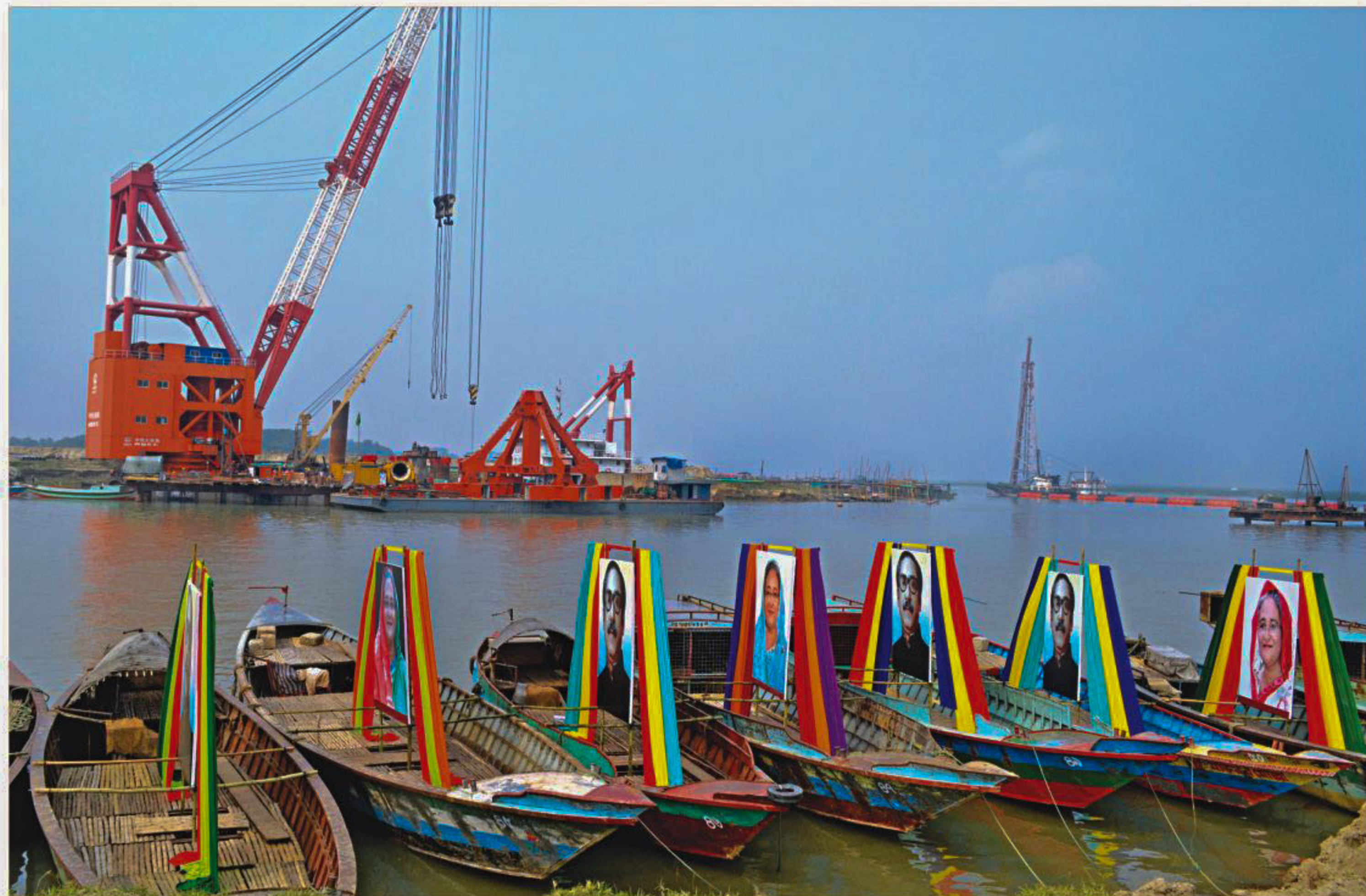
The inaugural site of the Padma bridge at Mawa has been decorated with portraits of Bangabandhu Sheikh Mujibur Rahman and Prime Minister Sheikh Hasina set on boats. The photo was taken yesterday.
