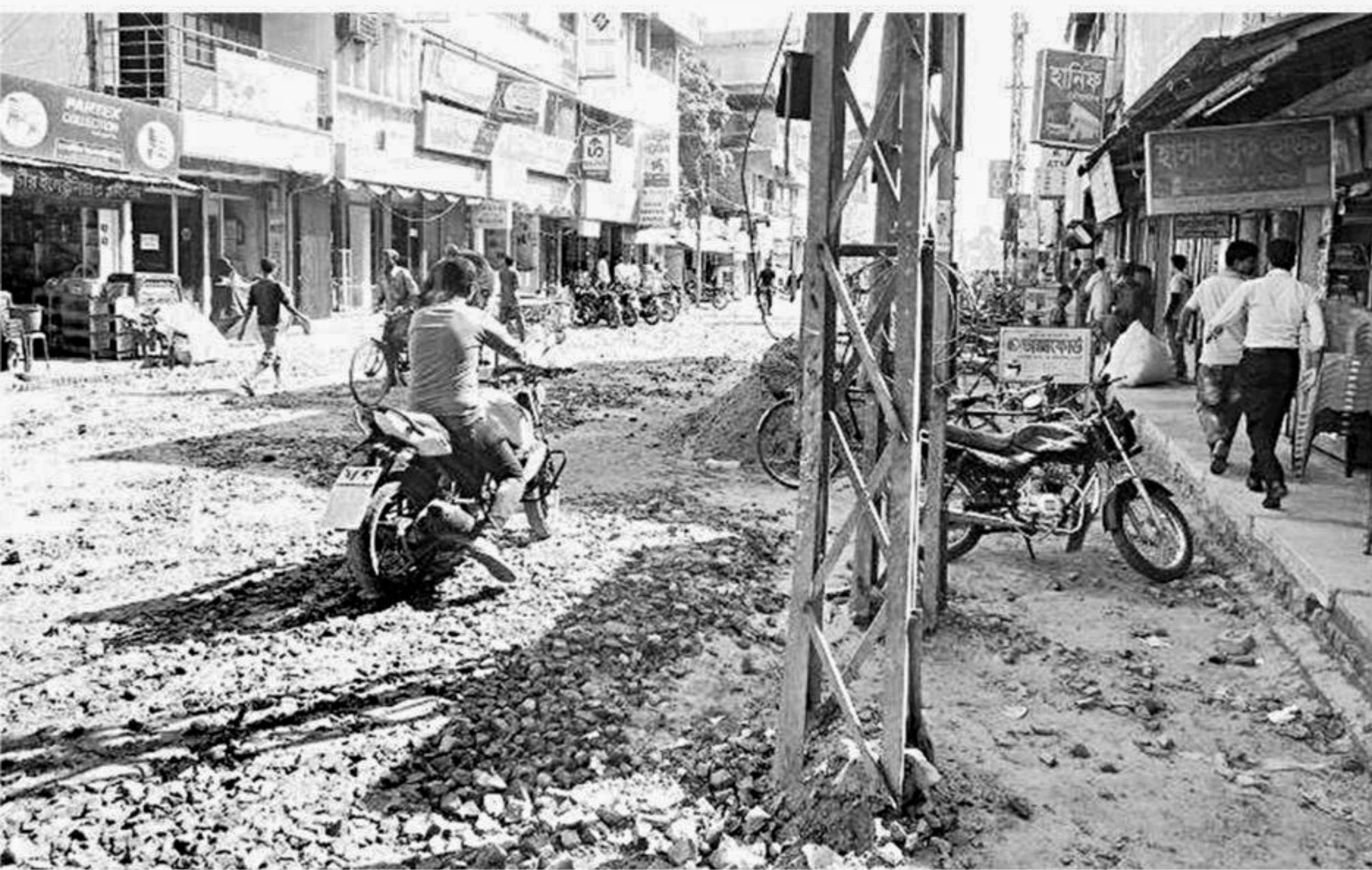
Road expansion work goes on, keeping electric poles over three feet inside, making futile the initiative to ease traffic congestion on Shaheed Dr Zikrul Huque Road in Saidpur municipality under Nilphamari district.
