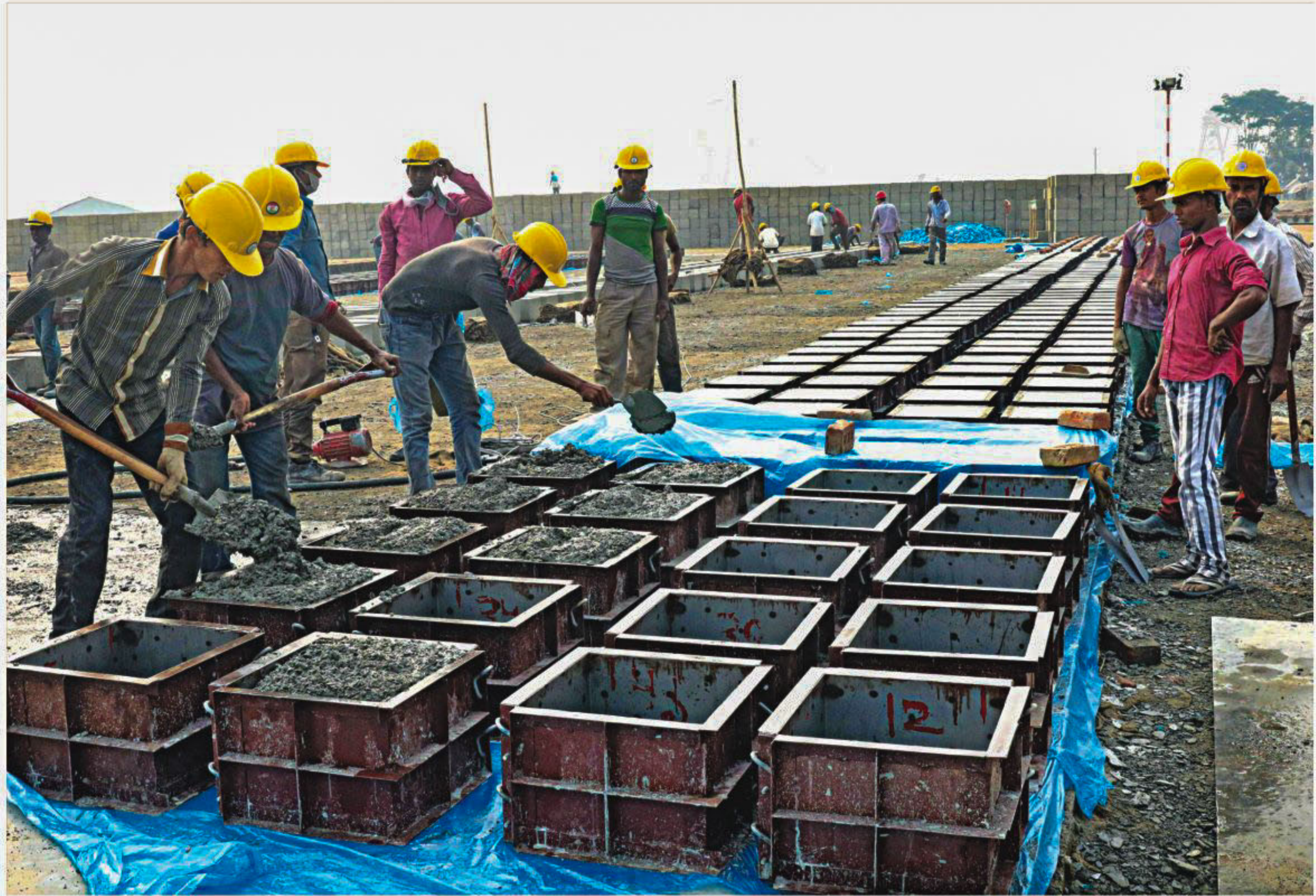
Concrete blocks are being made on the bank of the Padma at Mawa. Thousands of such blocks will be used in river training for construction of the Padma bridge. The photo was taken recently.
